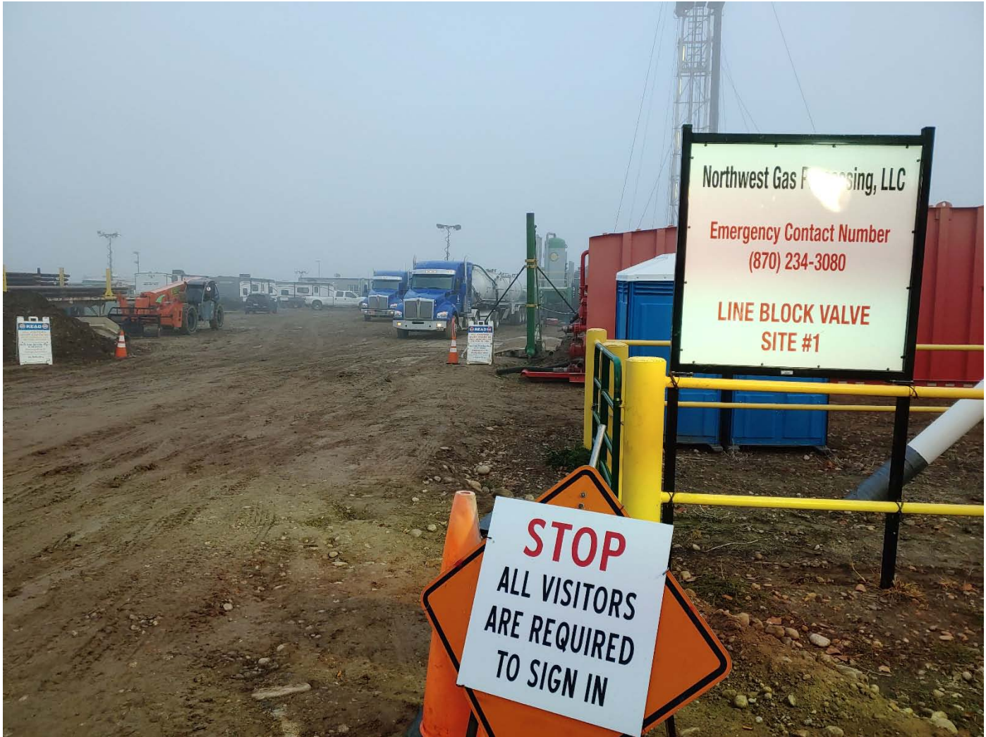
Harmon gathering line riser and block valve, entrance to Fallon #1-11 well pad looking N. from Killebrew Rd.
