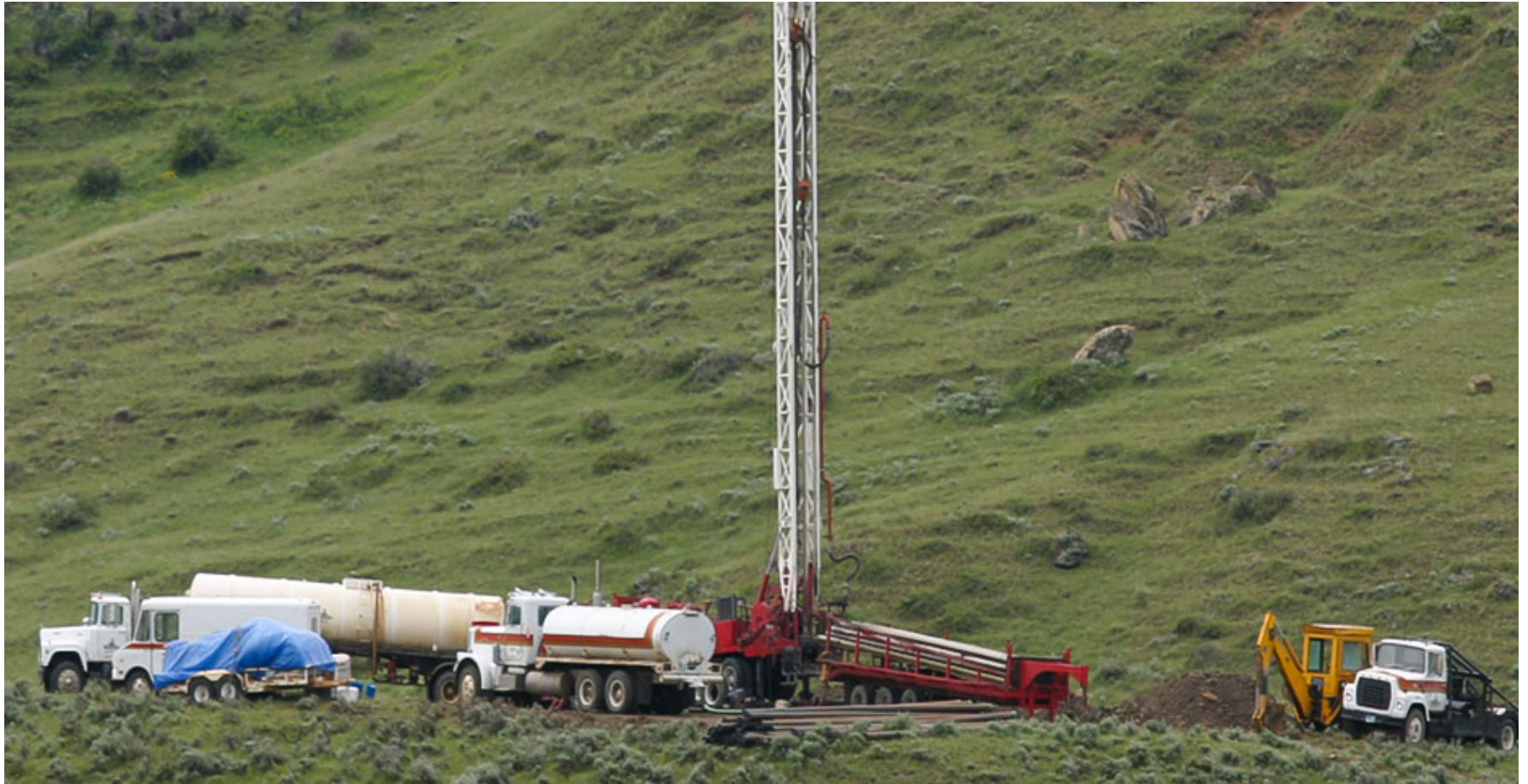
A coalbed methane well site. Montana Department of Natural Resources & Conservation
