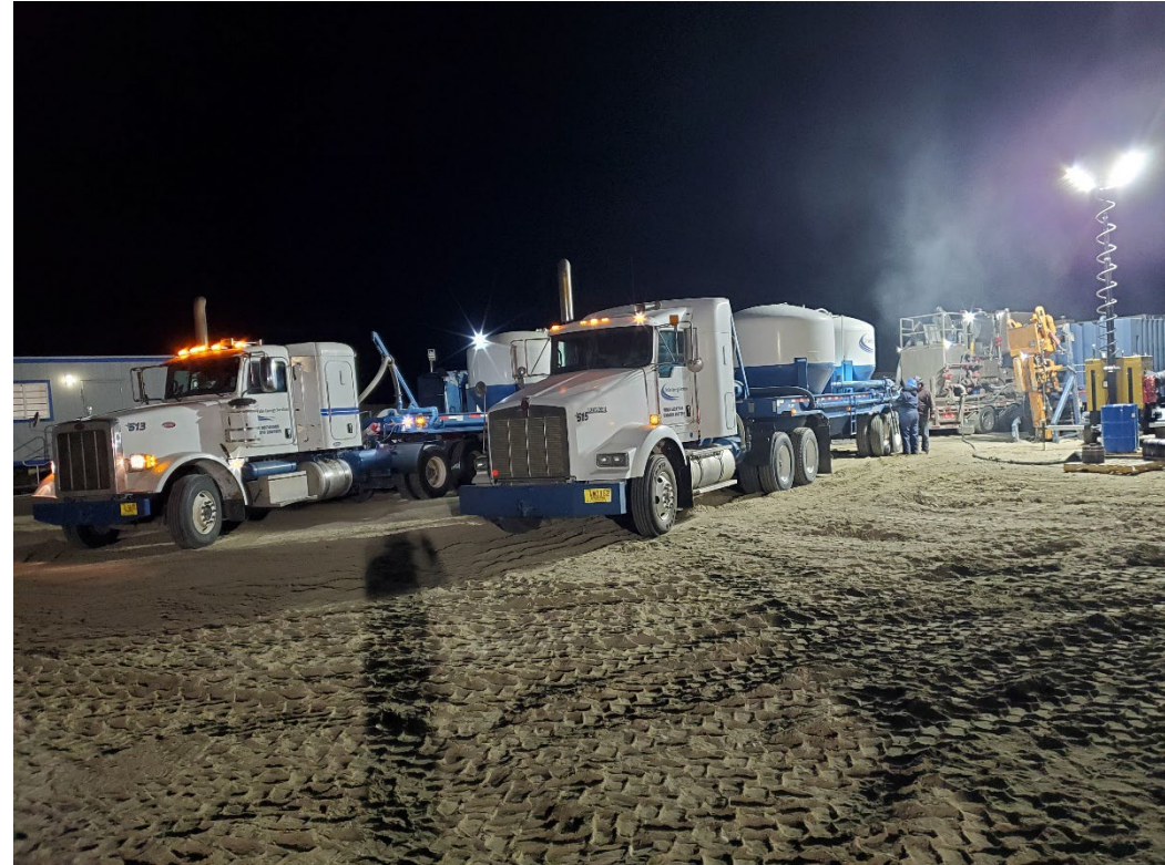
IDL on site to witness surface casing operations on the Twin Peaks #1W stratigraphic test, Canyon County, November 2025. Photo courtesy J. Thum
