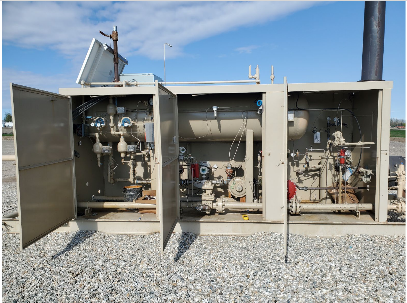
Interior Irvin #1-19 separator unit.
