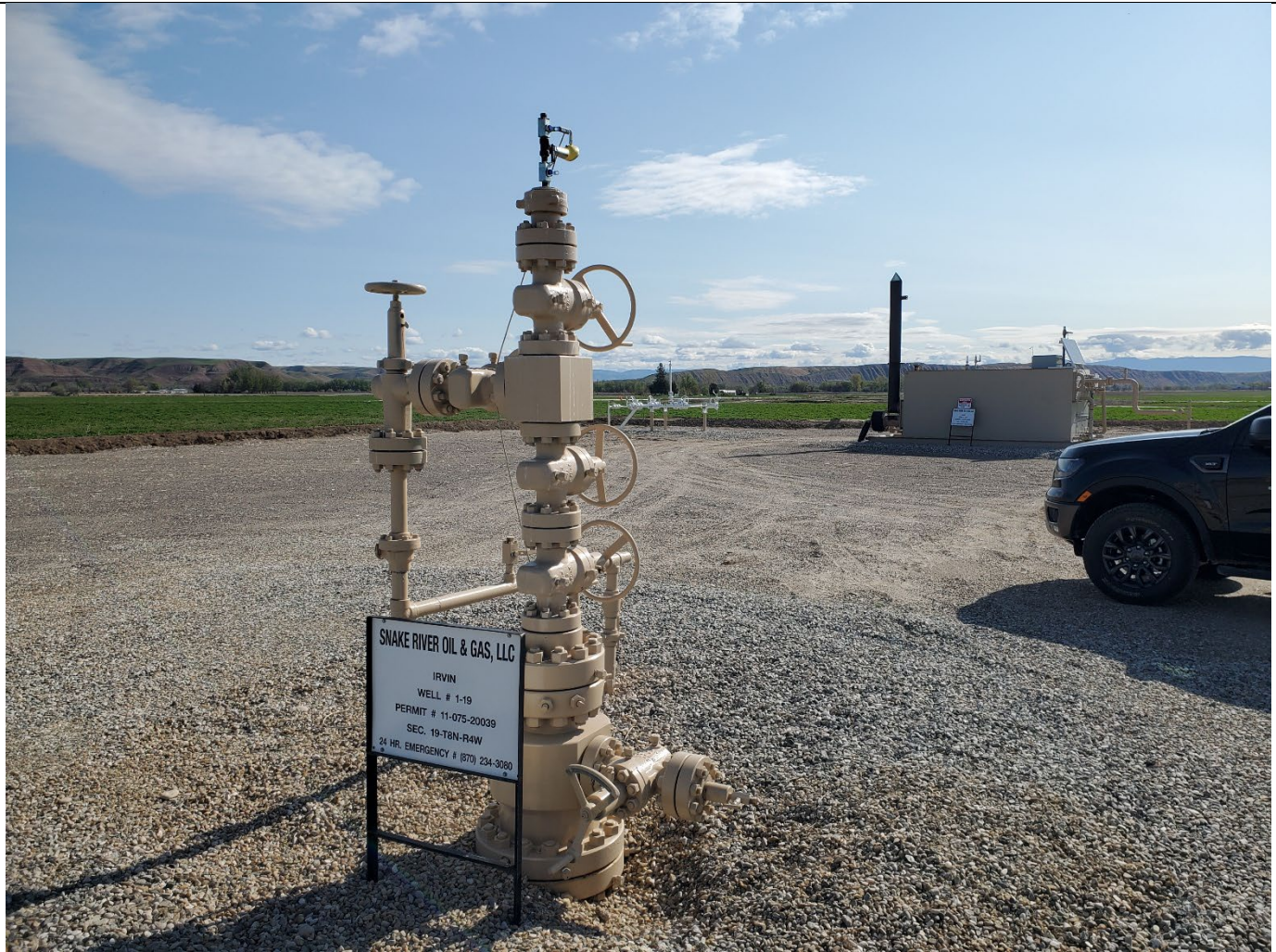
Wellhead left foreground with separator right background. Gathering riser center background. View is northeast.
