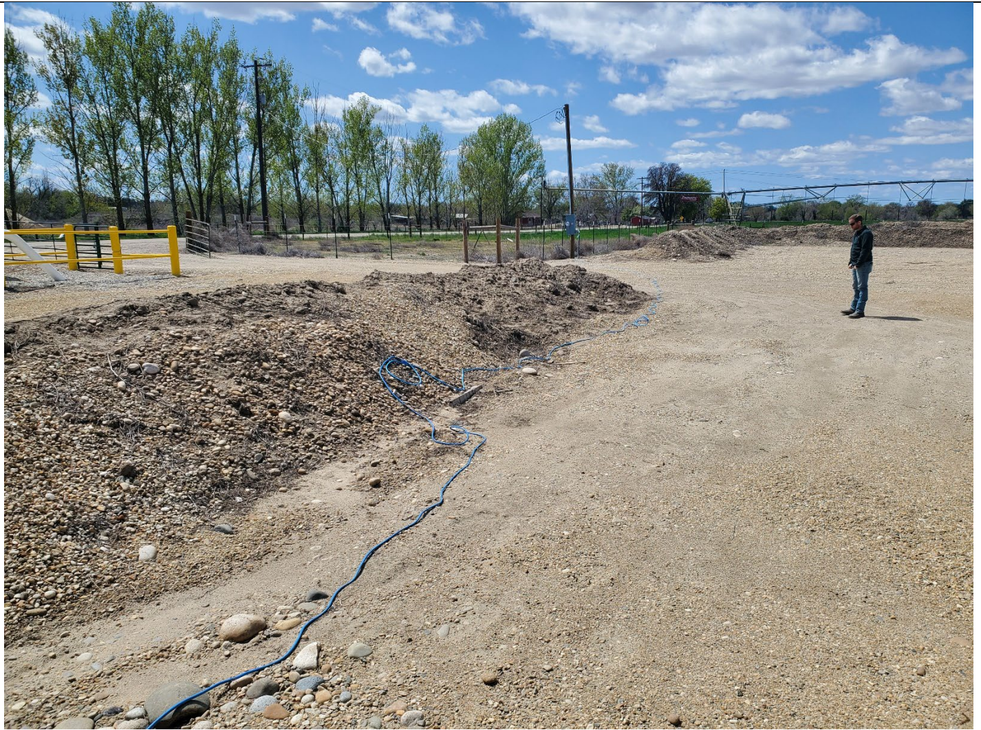
Blue extension cord as temporary power from separator unit to electric service box at pad gate.
