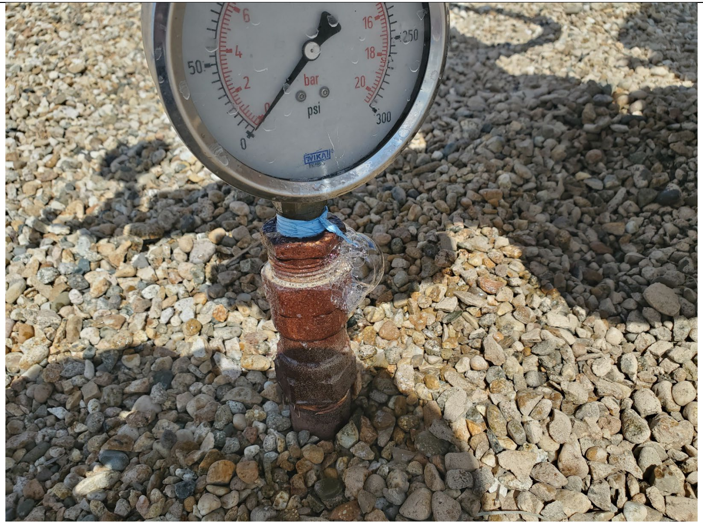
Analog pressure gauge for surface casing with small leak. Note pressure indicated as 0 PSI.
