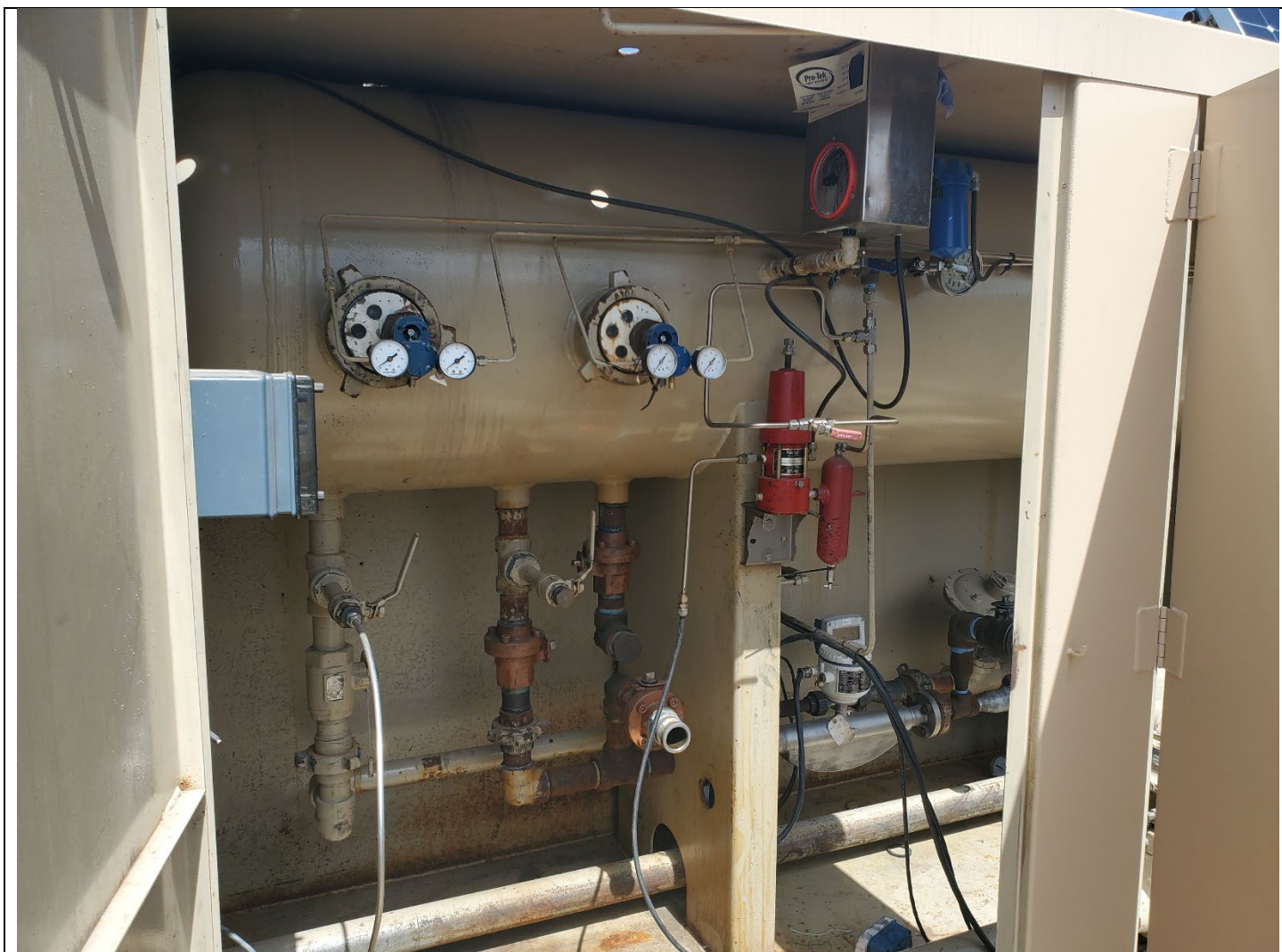
Left side interior of separator unit, coriolis flow meter at lower right.
