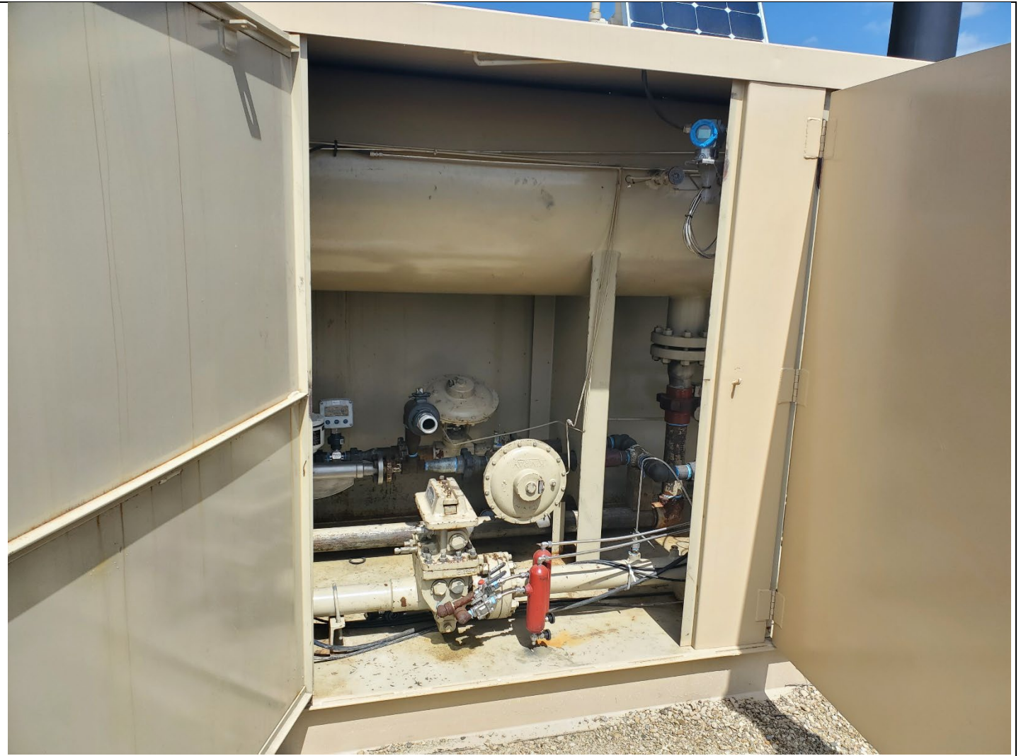
Right side interior of separator unit.
