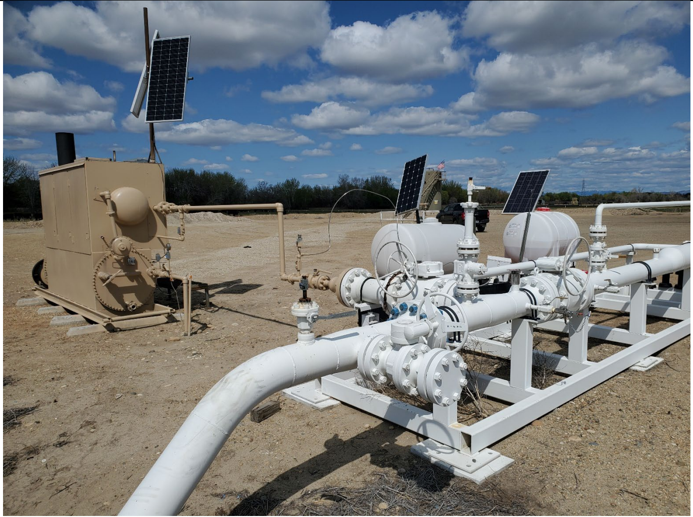
Gathering line riser, pig launcher far right. Wellhead and produced water tank rear center, separator at left. View is northwest.
