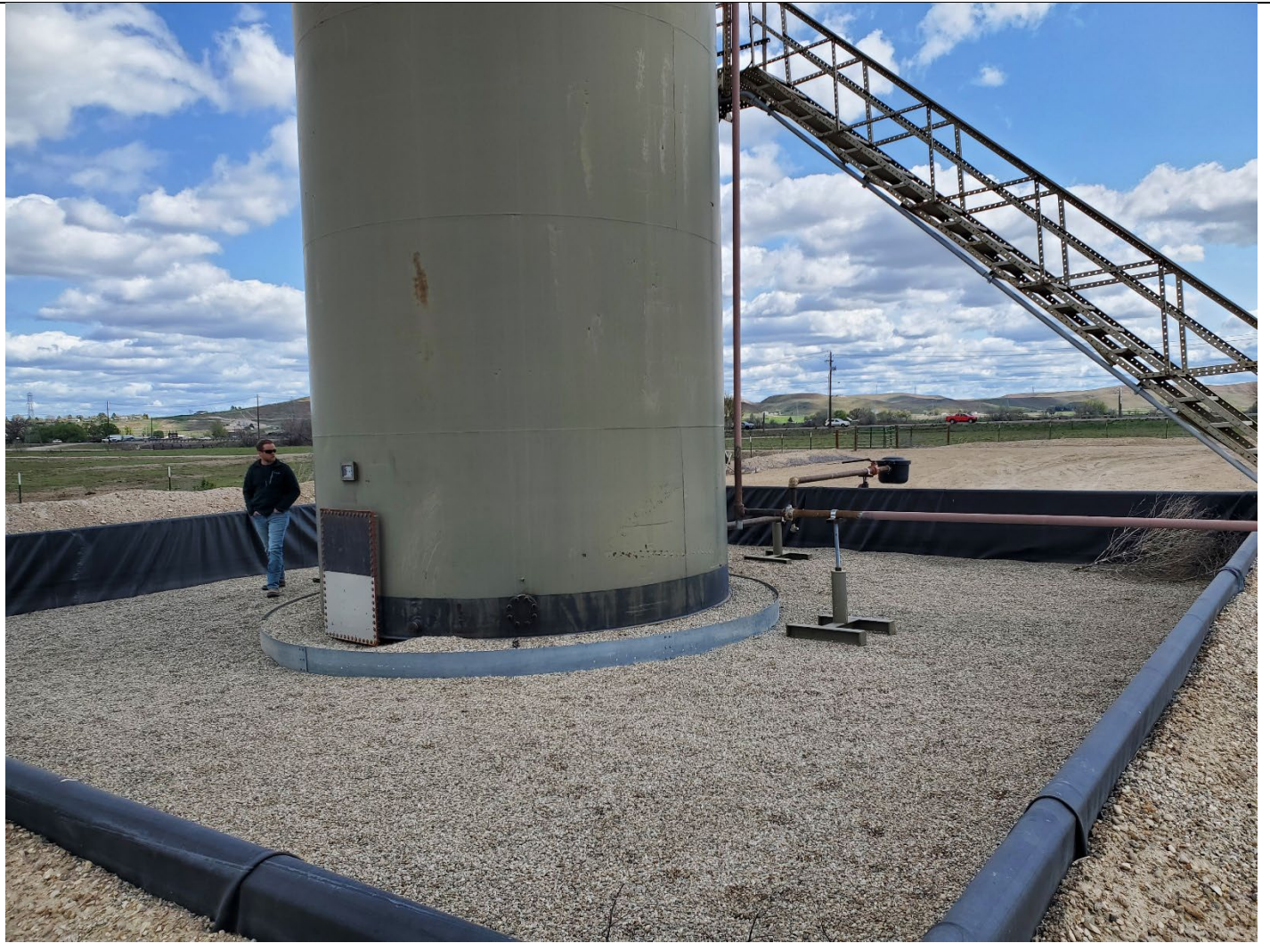
400 bbl produced water tank and containment berm. View is northeast.
