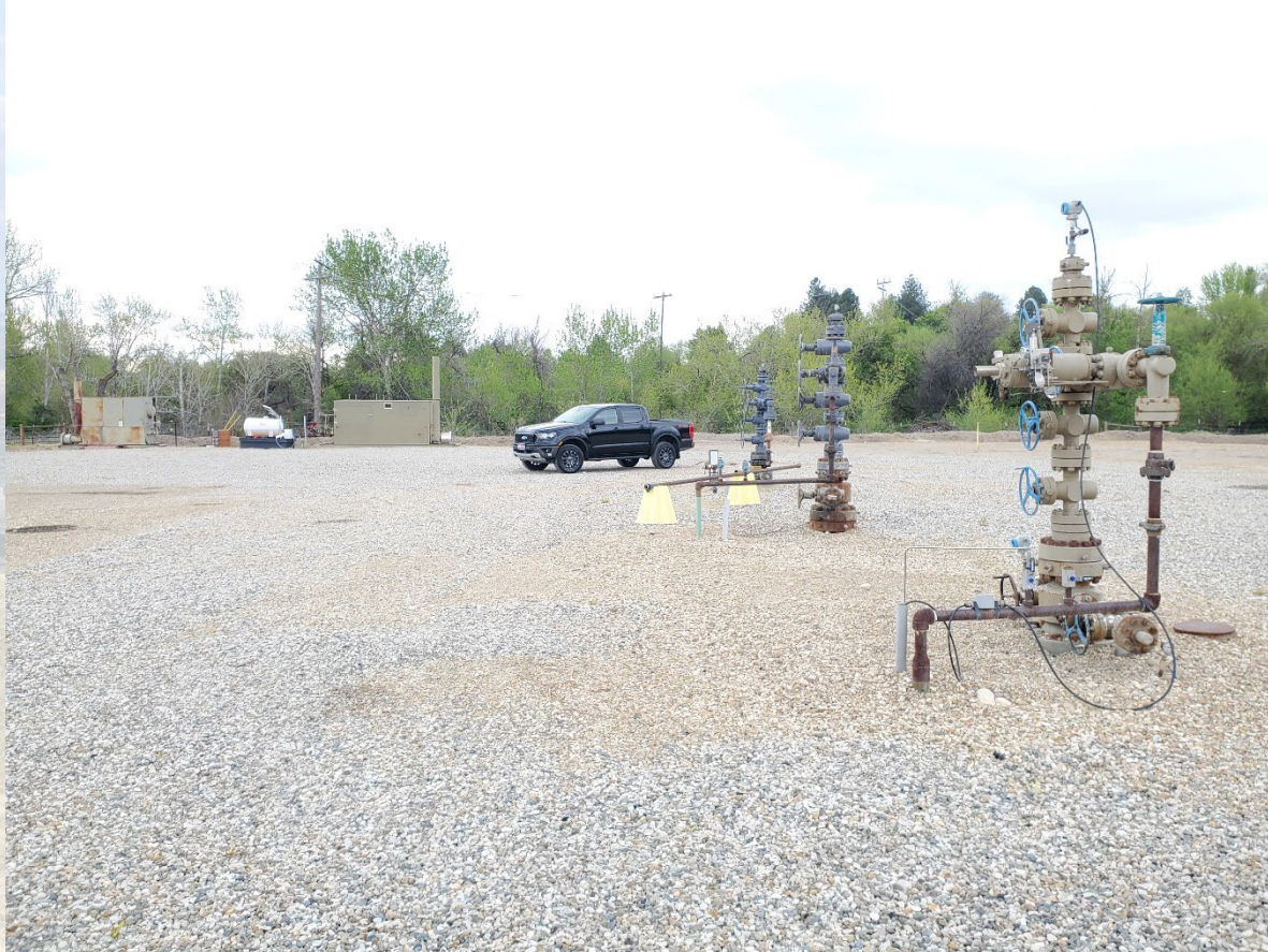
CENTER TO RIGHT – BARLOW #3-14, BARLOW #2-14, AND BARLOW #1-14 WELLHEADS APRIL 2024 PHOTO COURTESY J. THUM
