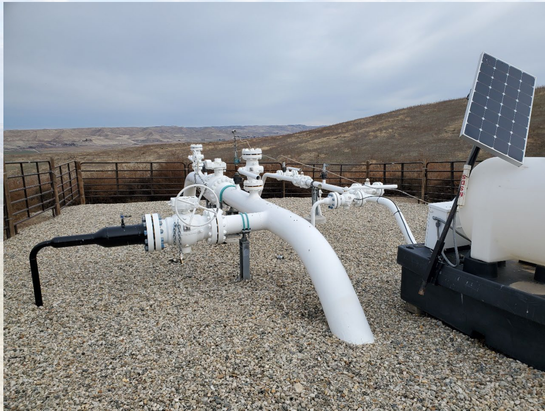
DJS #1-15 RISER LOOKING NORTH TOWARDS LITTLE WILLOW GATHERING FACILITY, NOVEMBER 2023 PHOTO COURTESY J. THUM
