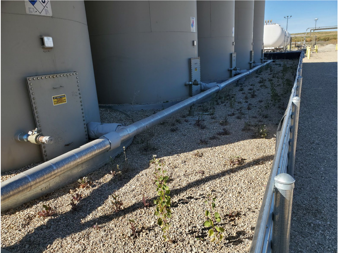
Vegetation within the condensate tank dike, west side of facility. View is north-northwest.
