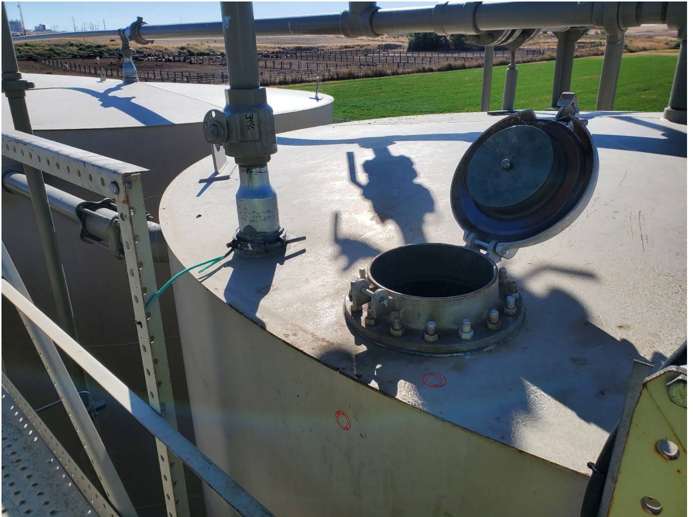
Condensate tank vent lid in open position, northwestern-most condensate tank. View is southwest.
