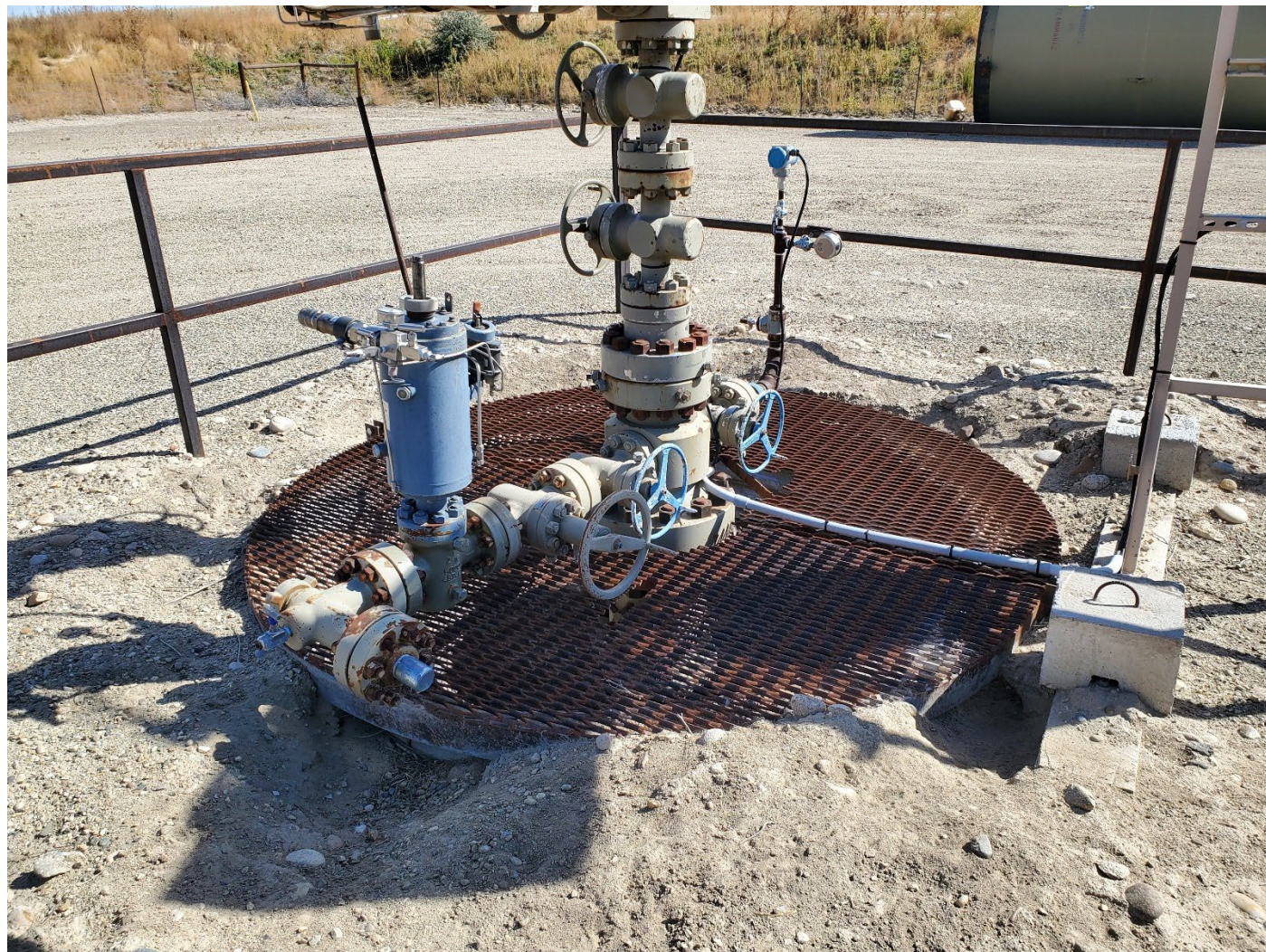
Wellhead and conductor showing apparent animal burrowing activity (not new). View is East.
