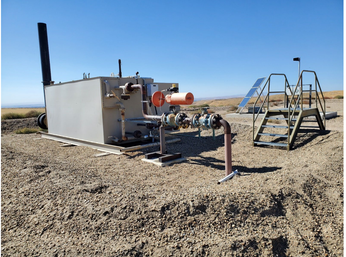
Separator unit and access ladder over retention barrier. SCADA system solar panel in background. View is West.
