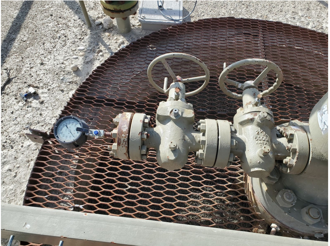
View of production casing gauge and cellar on UT completion side.
