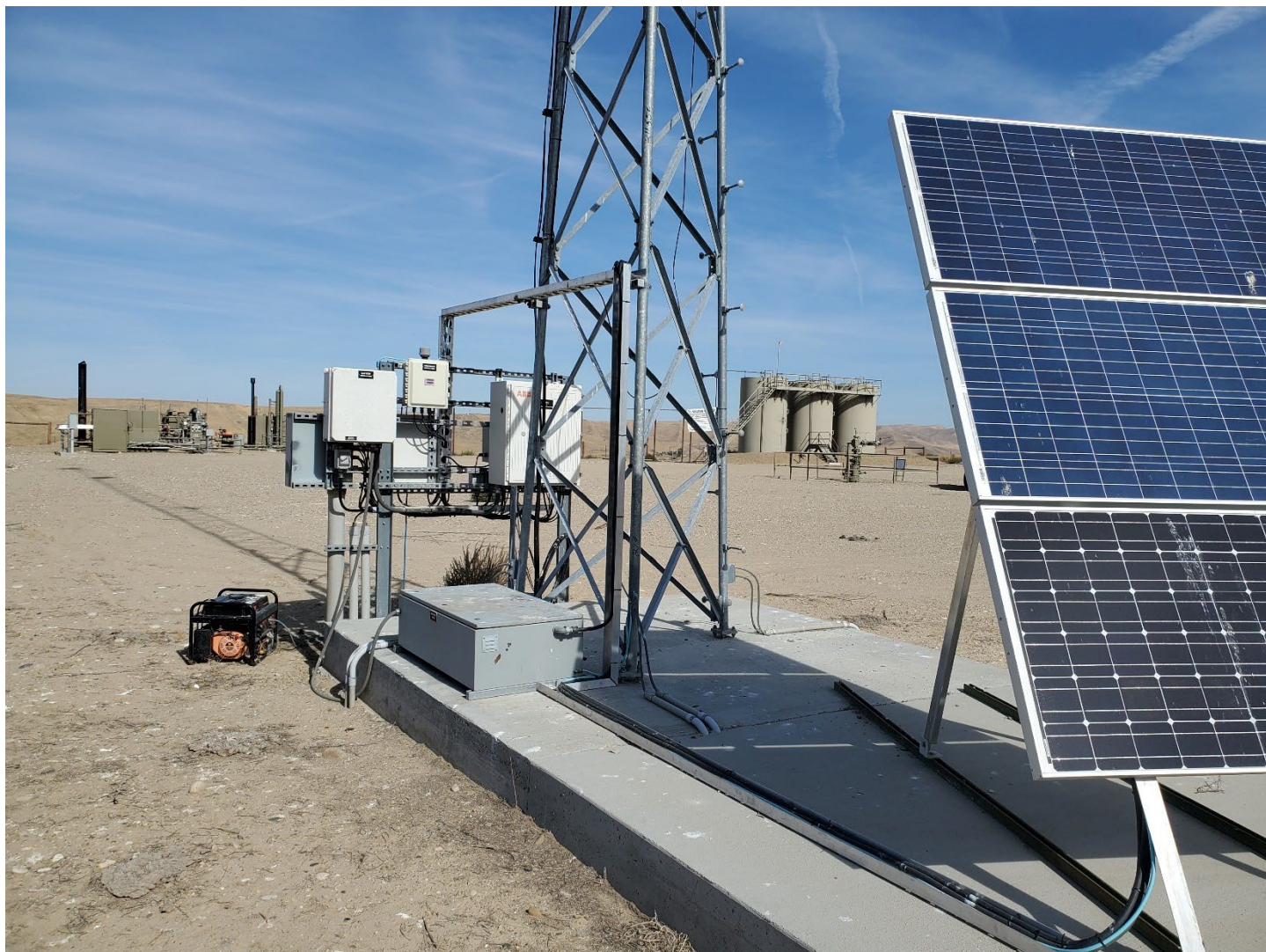
SCADA system and solar panels (foreground), separator unit (left background), tank battery and wellhead (center background). View is north.
