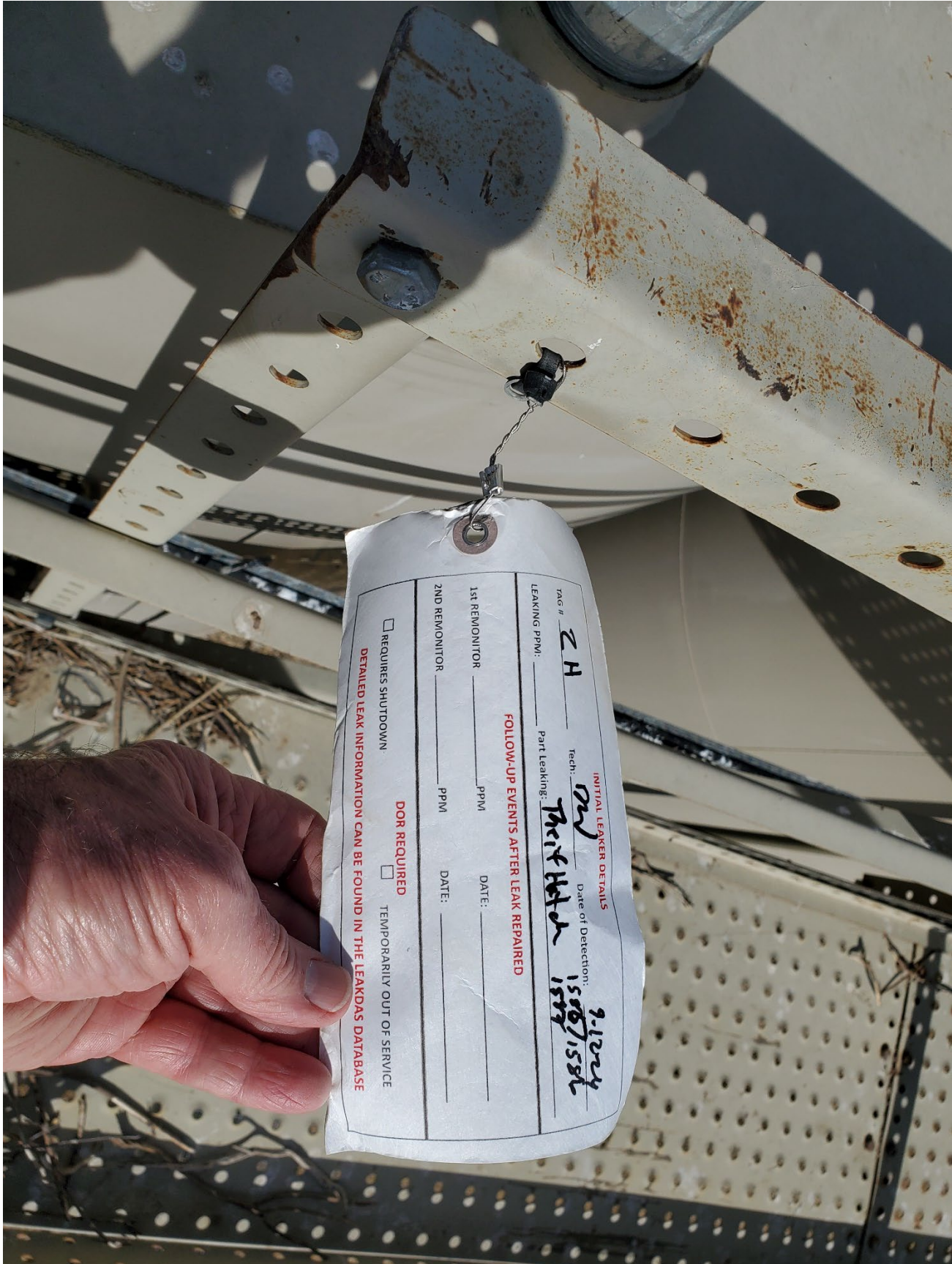
Thief hatch leak tag dated 9/12/2024, southwesternmost produced water tank.
