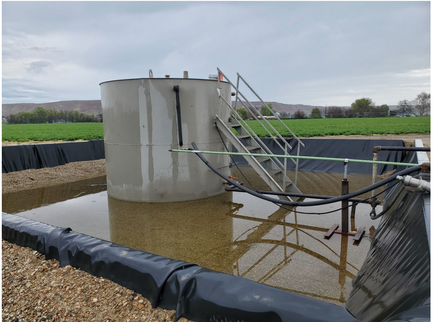
Photo #115231: Produced water tank and containment dike, view northeast. Leak tag at top of ladder, top right side of water tank (tag not inspected). Approximately 9 inches of water in containment dike from recent rain.
