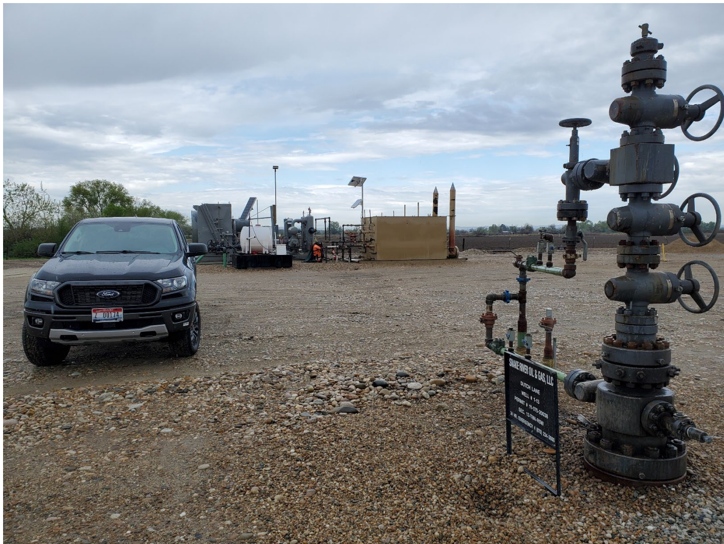
Photo 114636: Wellhead to right, separator at center rear, compressor unit to left rear behind inspection vehicle. View is west.
