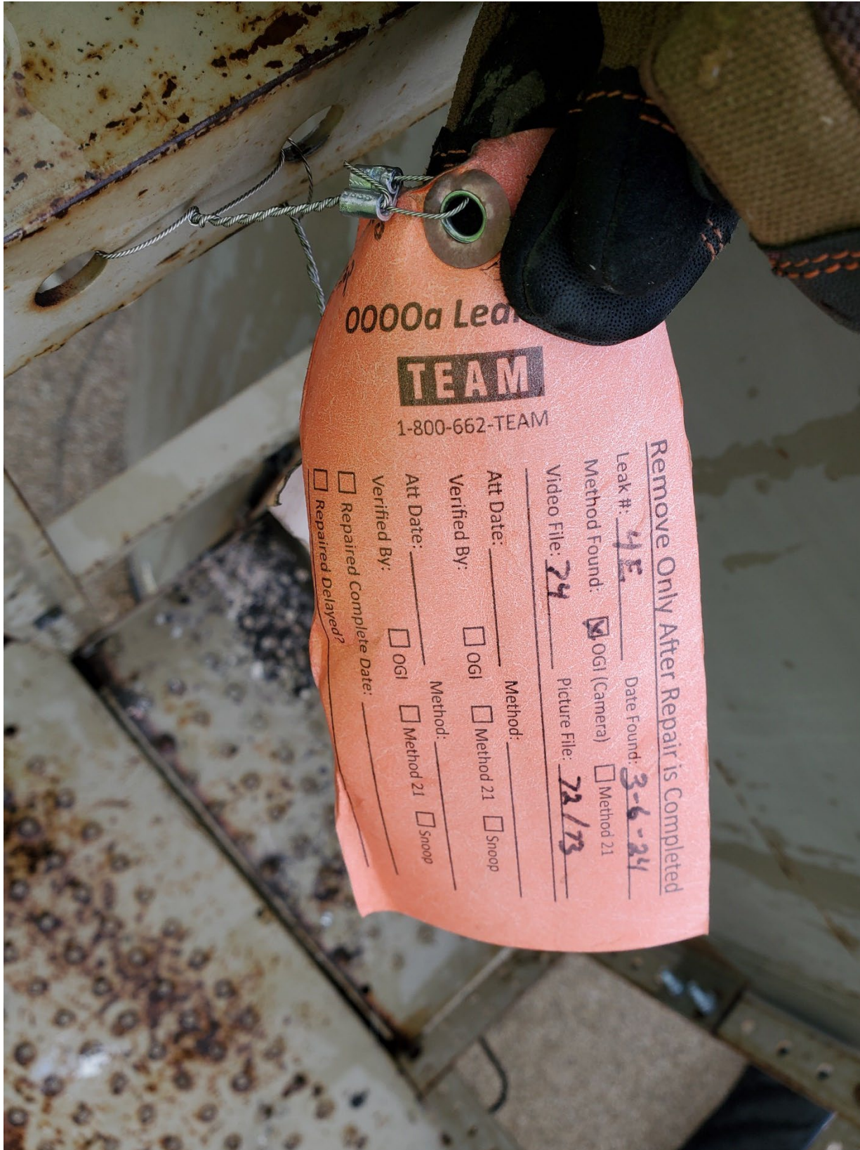
Photo #111330: Leak tag on top of produced water storage tank.
