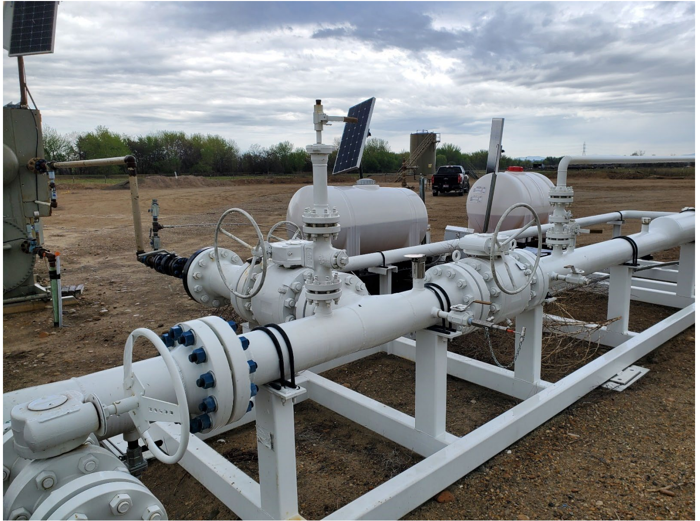
Photo 110846: Pig launcher and chem tanks, separator on left. View northwest.
