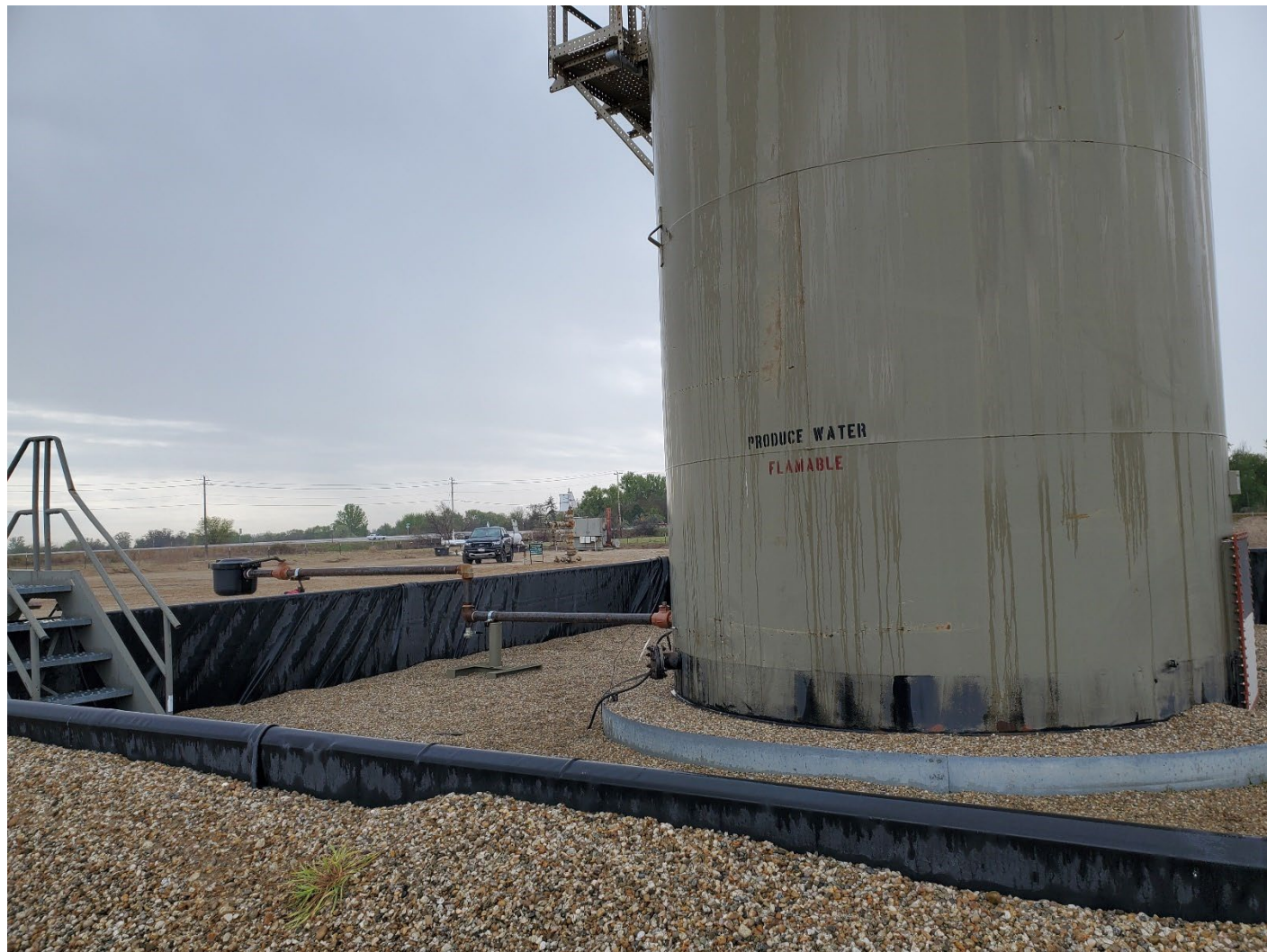
Photo 111026: Produced water tank and containment dike. View is SE.
