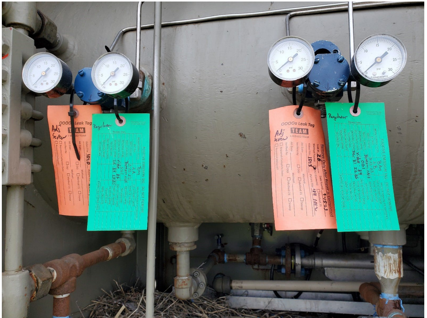
Photo 110604: Leak tags on pneumatic valves in separator. Operator is in the process of converting valves to nitrogen-actuated to comply with new 2024 EPA requirements.
