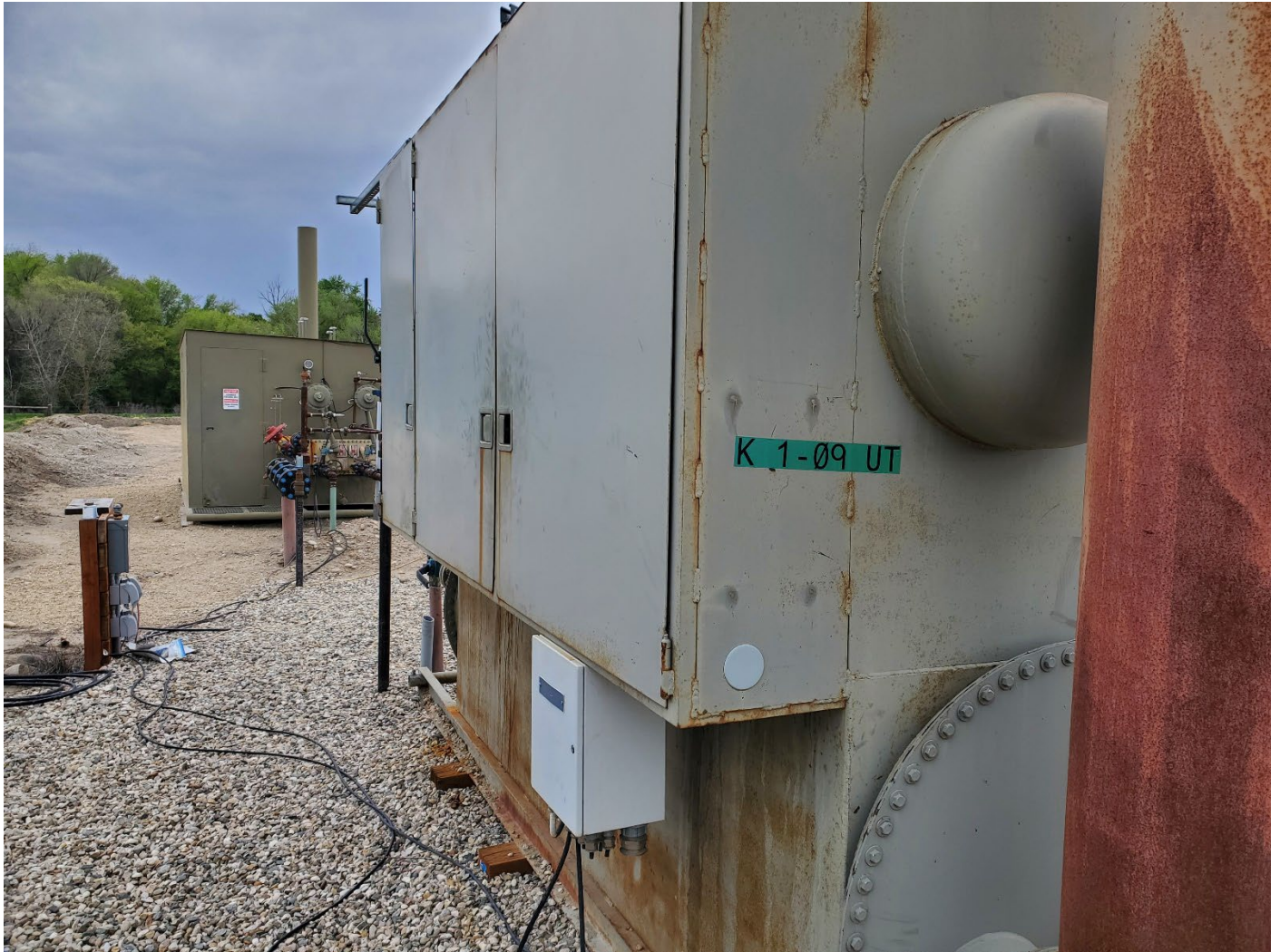
Photo 094815: Barlow #3-14 separator unit recycled from Kauffman #1-9 UT. Dual separator for Barlow #1-14 and #2-24 at left background. View is SW.
