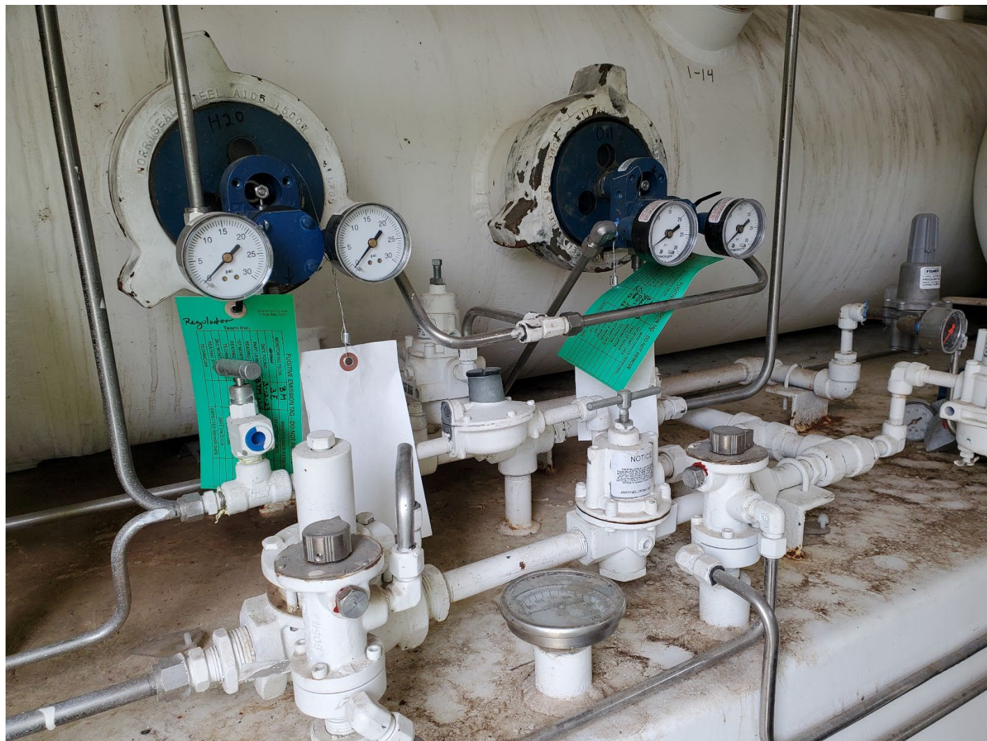
Photo 095408: Leak tags on dual separator unit from TEAM inspections. Operator is in the process of converting pneumatic valve systems to nitrogen-activated to comply with 2024 EPA emissions requirements.
