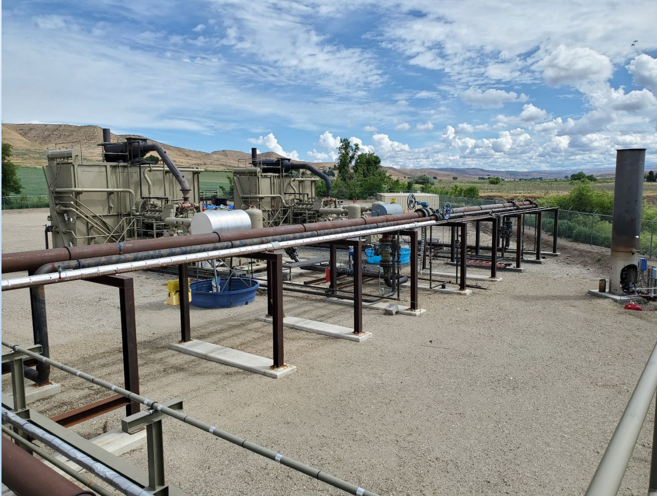
DUAL COMPRESSORS INSTALLED AT LITTLE WILLOW GATHERING FACILITY, JUNE 2023 PHOTO COURTESY J. THUM
