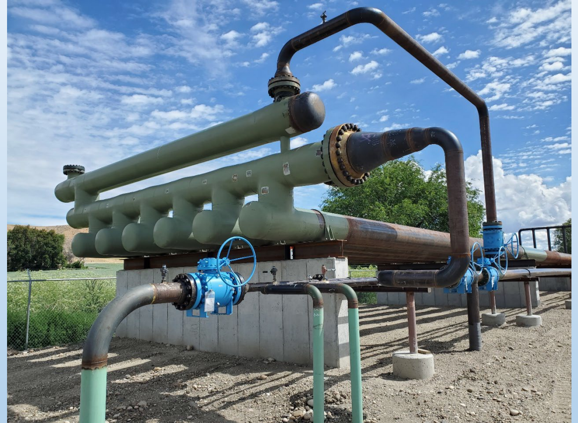
WESTERN END OF SLUG CATCHER FOR HANDLING PRODUCED LIQUIDS AT LITTLE WILLOW GATHERING FACILITY JUNE 2023 PHOTO COURTESY J. THUM
