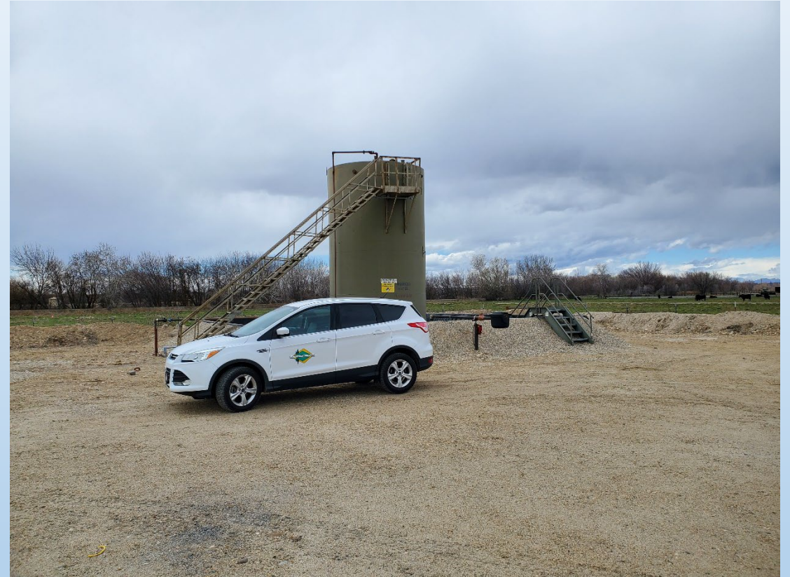
WATER TANK INSTALLATION INSPECTION ON THE FALLON 1-10 WELL PAD, APRIL 2023 PHOTO COURTESY J. THUM
