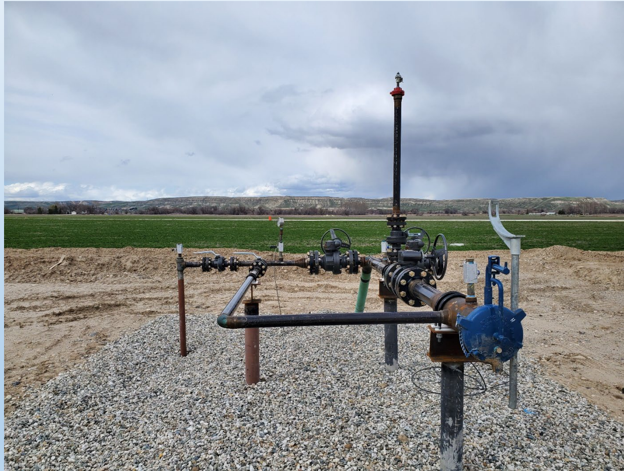
WELL FACILITIES INSTALLATION FOR THE IRVIN 1-19 WELL PAD, APRIL 2023 PHOTO COURTESY J. THUM
