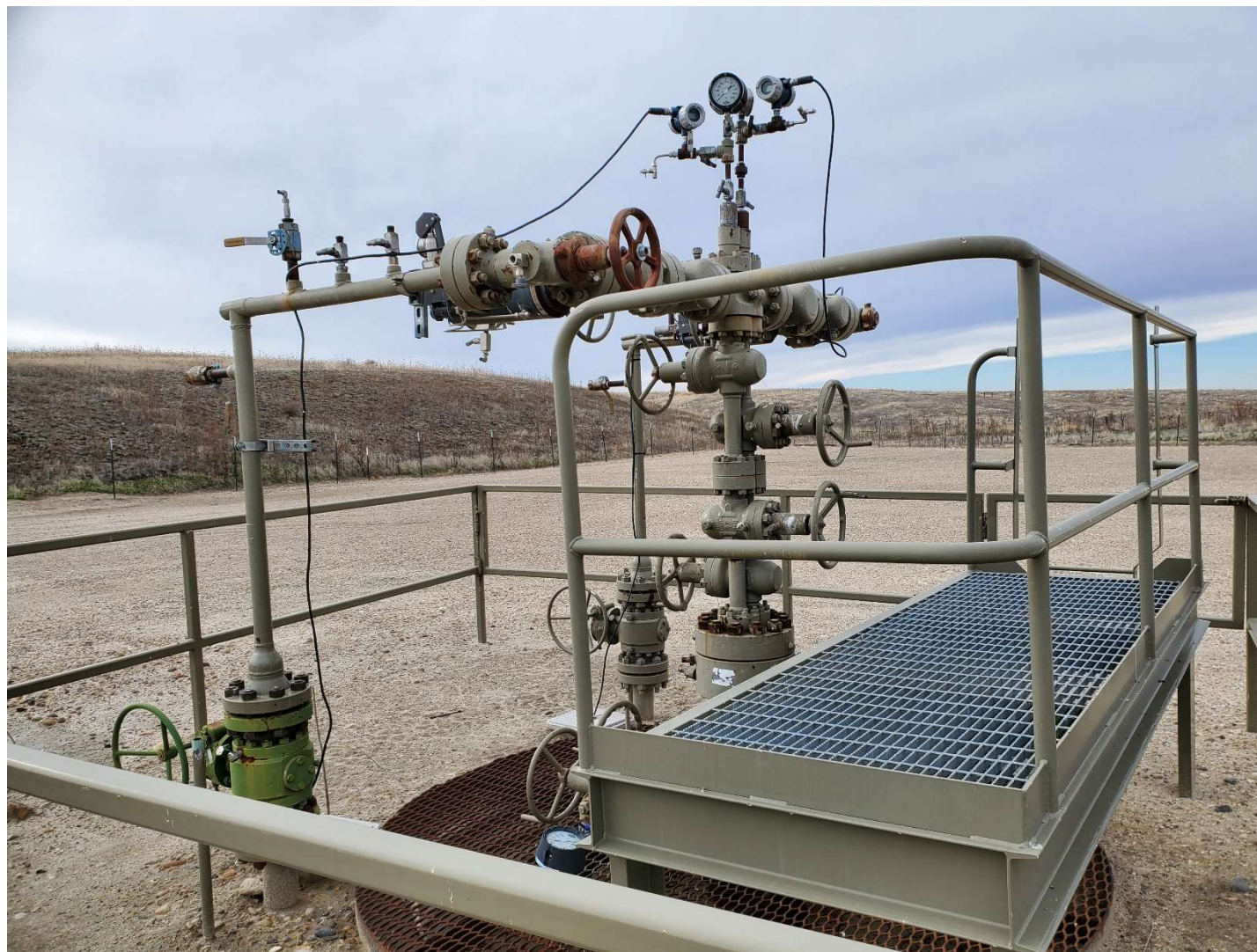
Wellhead showing pressure gauges installed on tree. View is Southwest.
