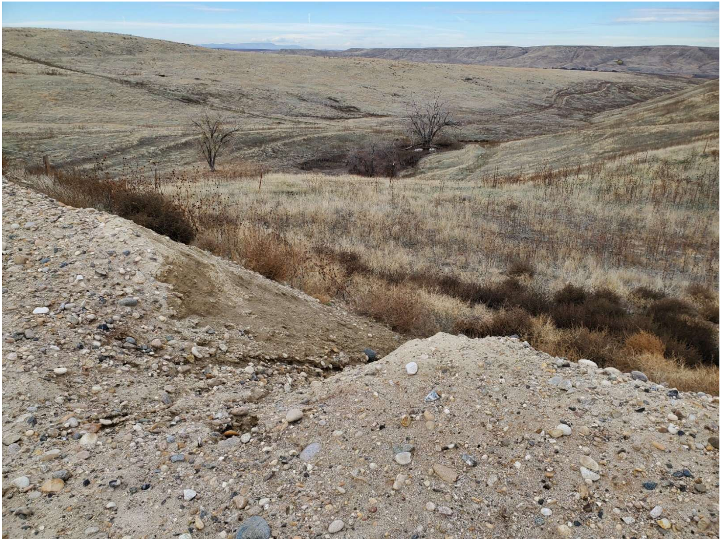
Well pad erosion on northwest perimeter. View is West.
