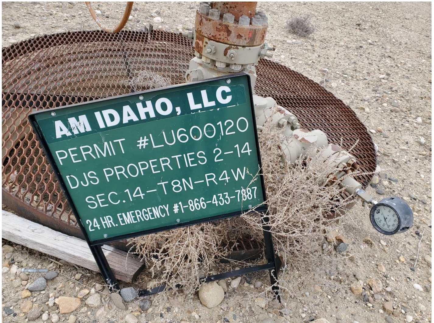
View of well head and open cellar, sign, and production casing analog pressure gauge.
