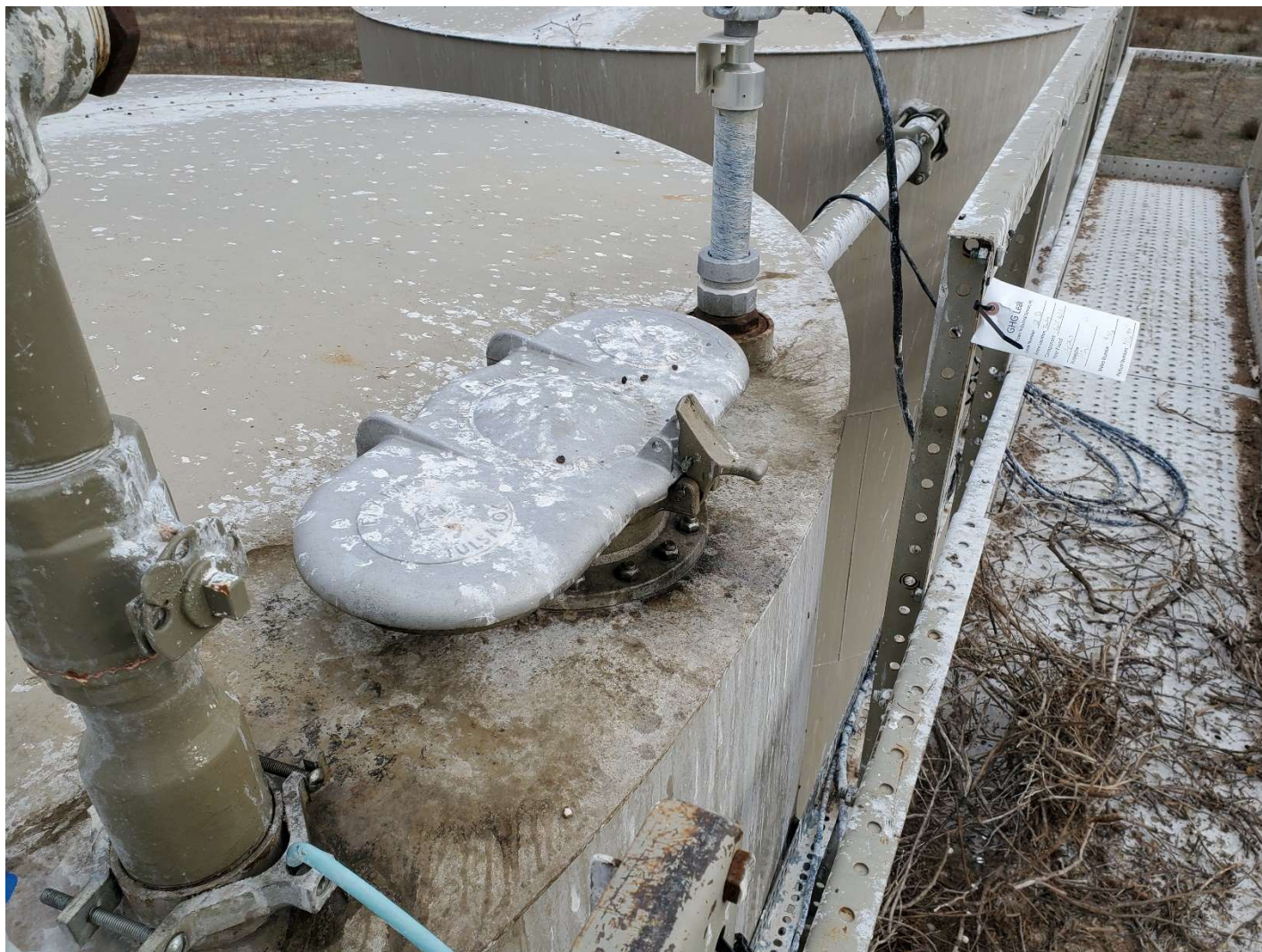
Leak tag attached at railing by thief valve on middle produced water tank.
