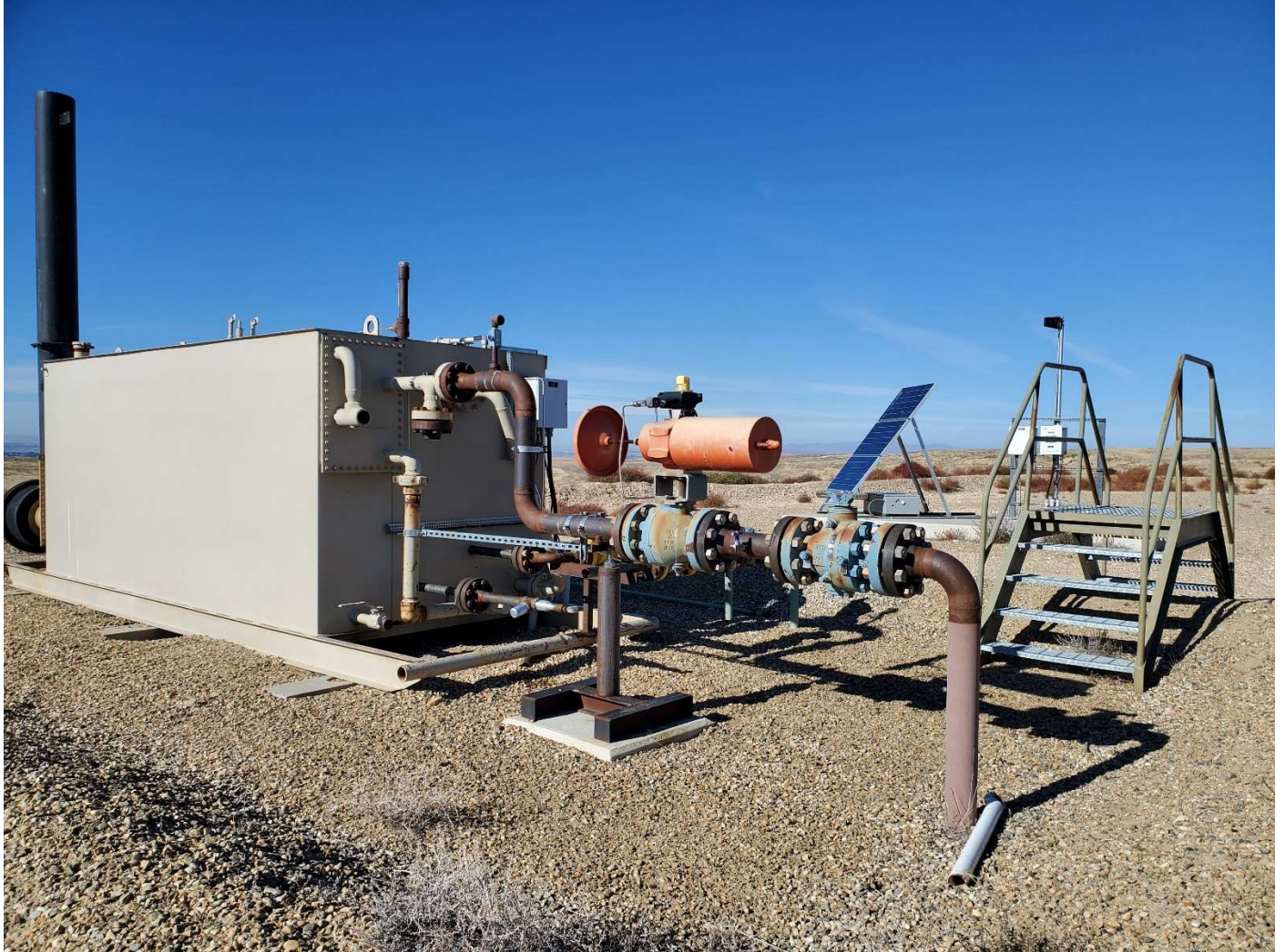
Separator unit with solar panels and control boxes in background. View is west.
