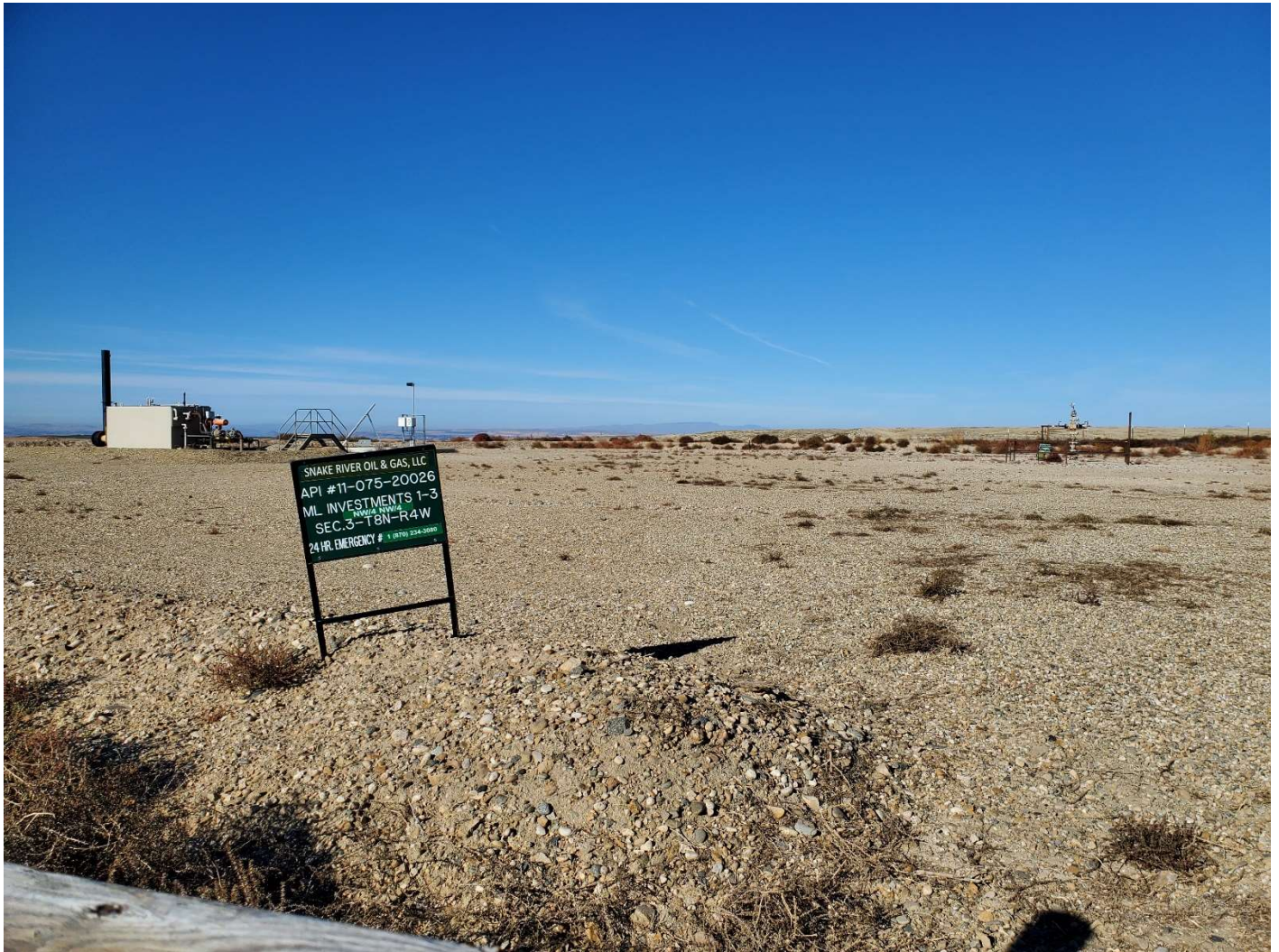
Pad overview, wellhead in right background, separator unit left background. View west.
