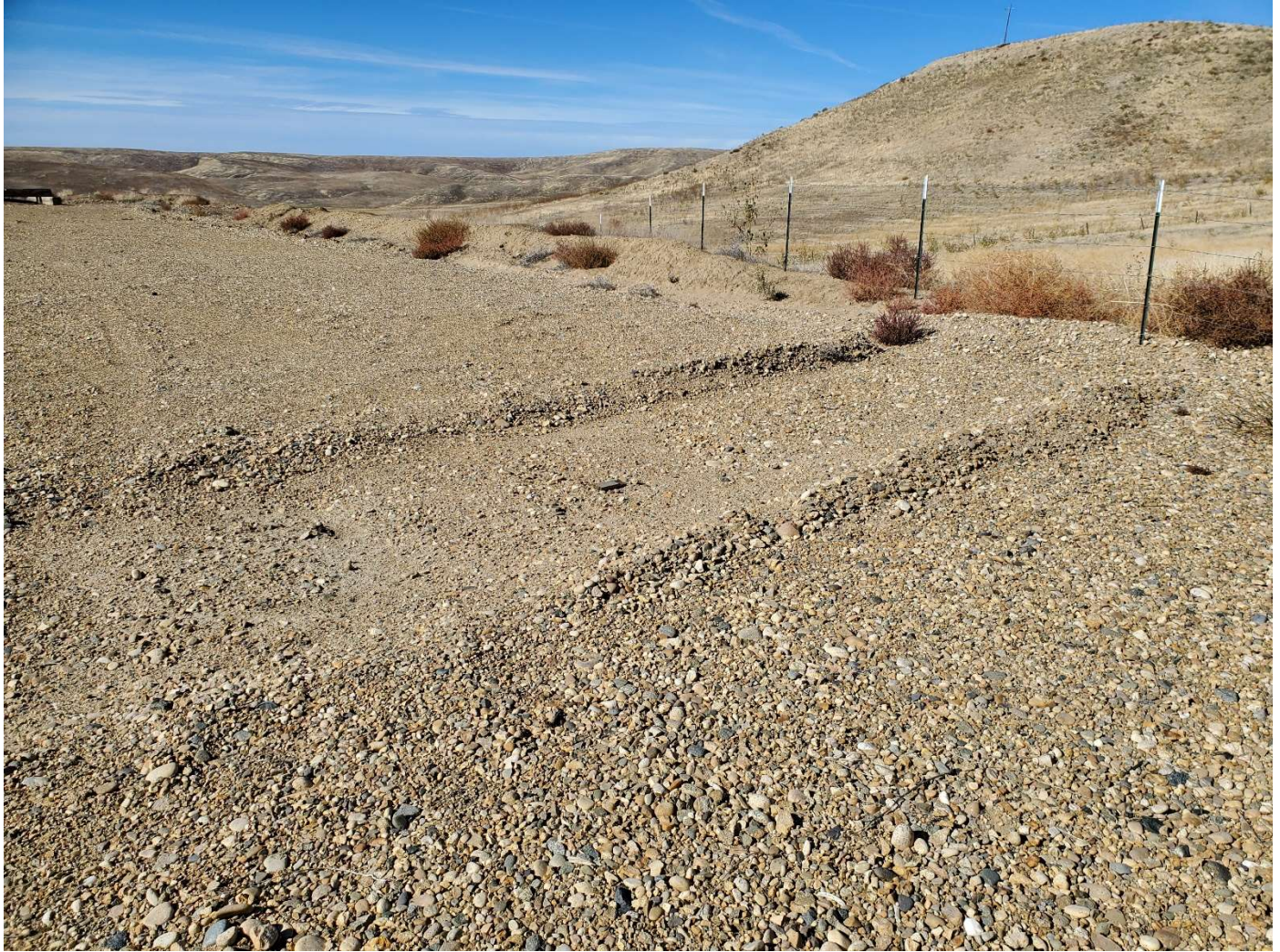
Constructed trench to prevent pooling snowmelt and runoff, northwest side of pad. View is west.
