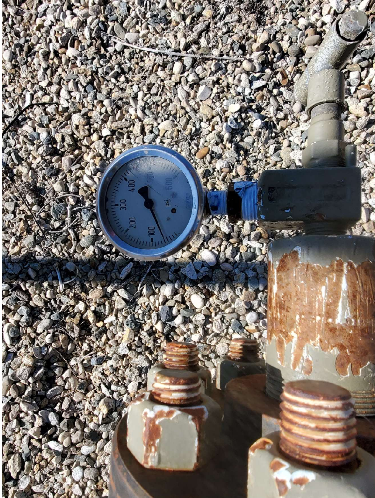
Production casing gauge
