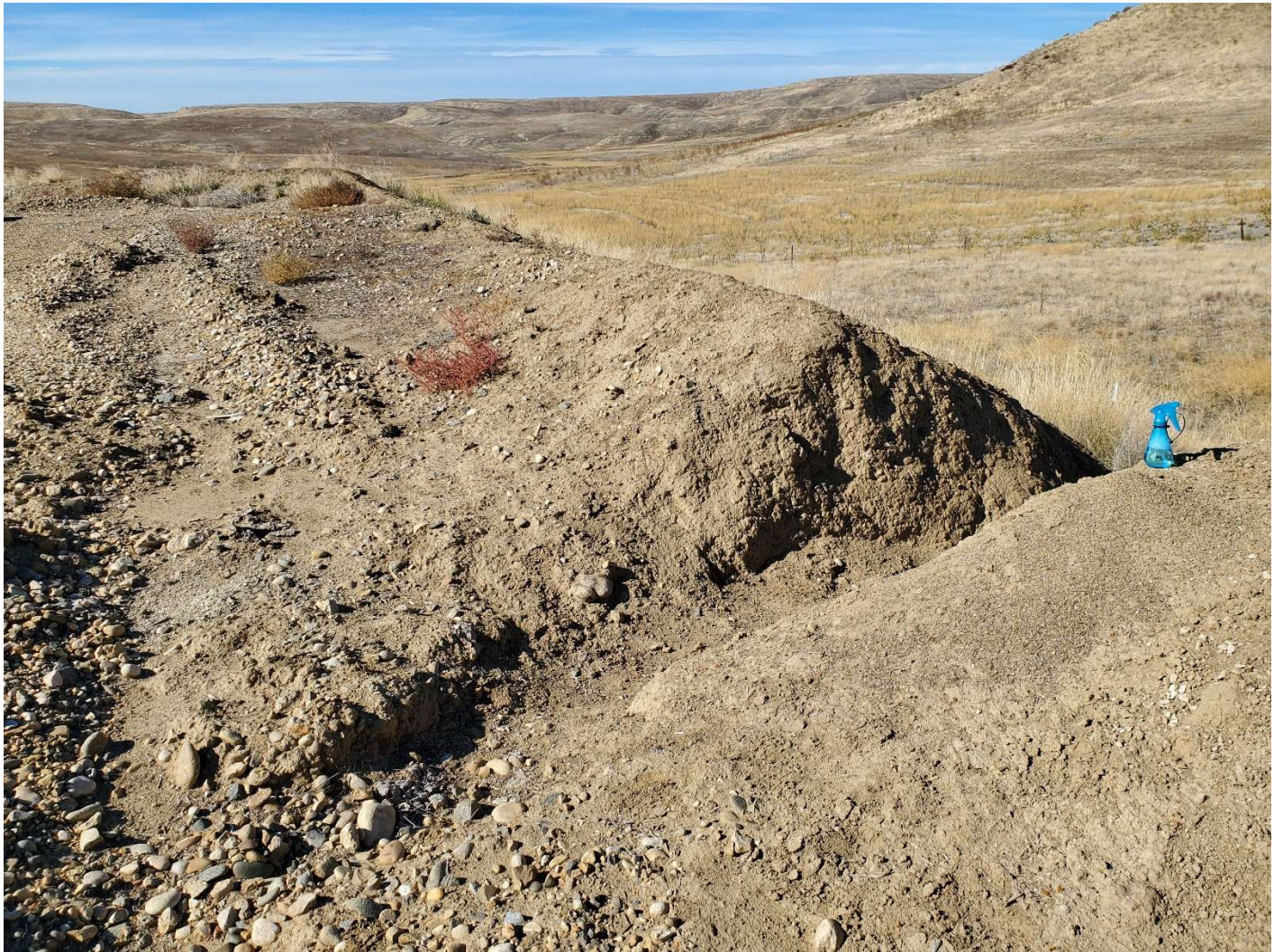
Constructed trench to prevent pooling snowmelt and runoff, northwest side of pad. View is west.
