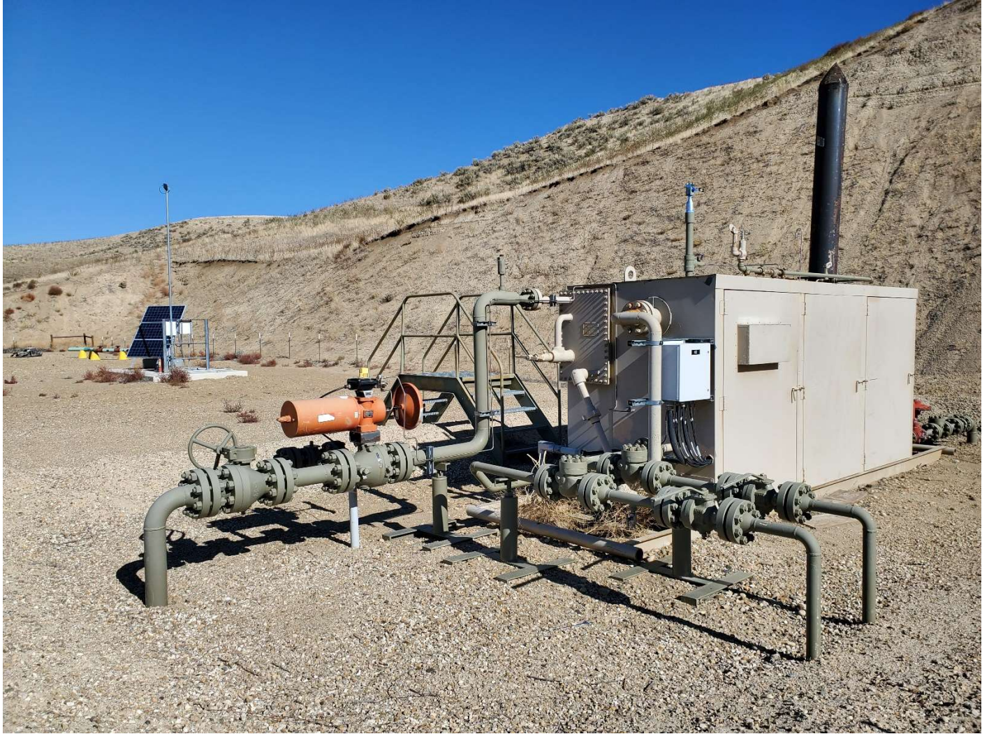
Separator unit looking north at cutbank. Solar array and control boxes in left background.
