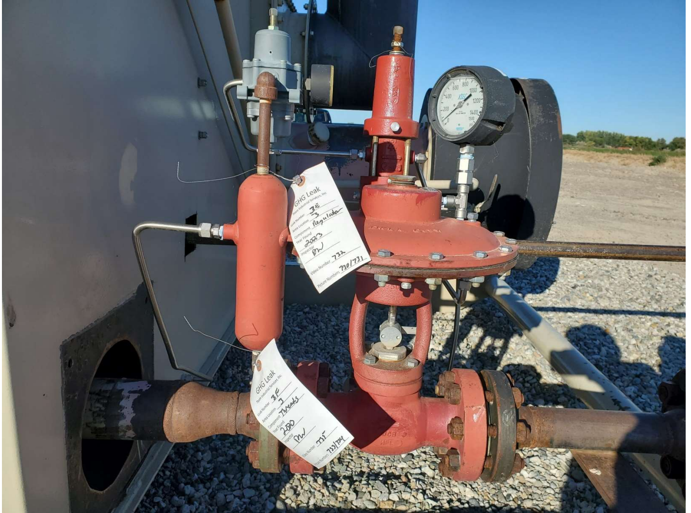
Leak tags on north exterior of separator unit.
