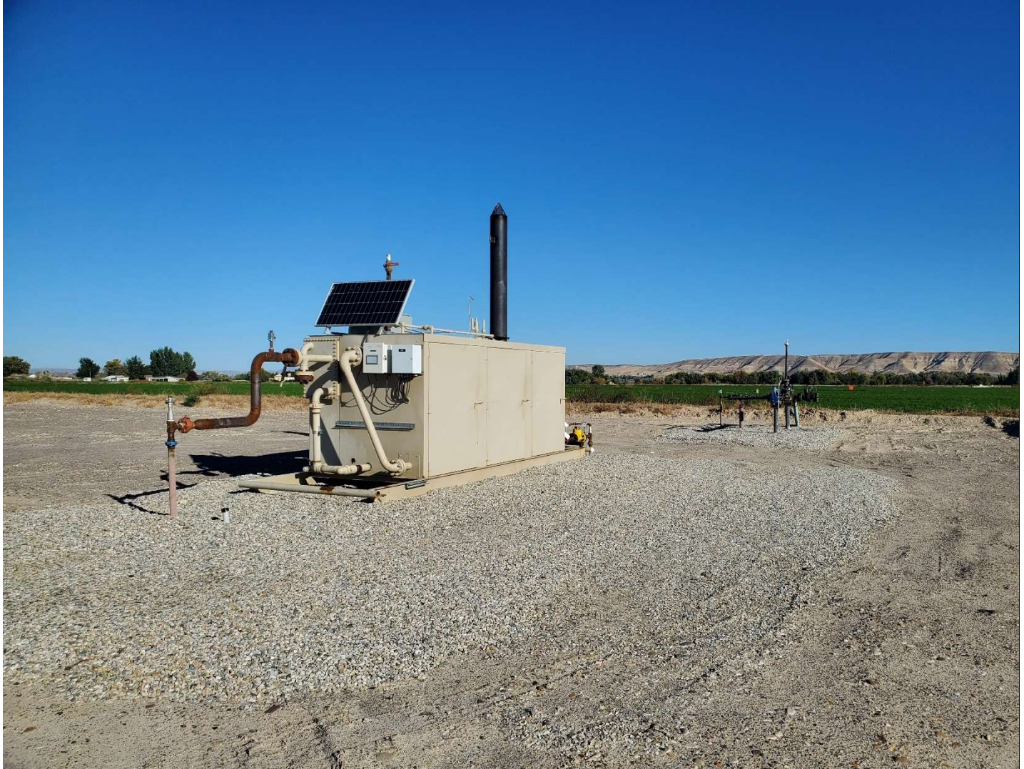
Separator Unit, northeast side of well pad looking NNW. Riser for gathering line to the right.
