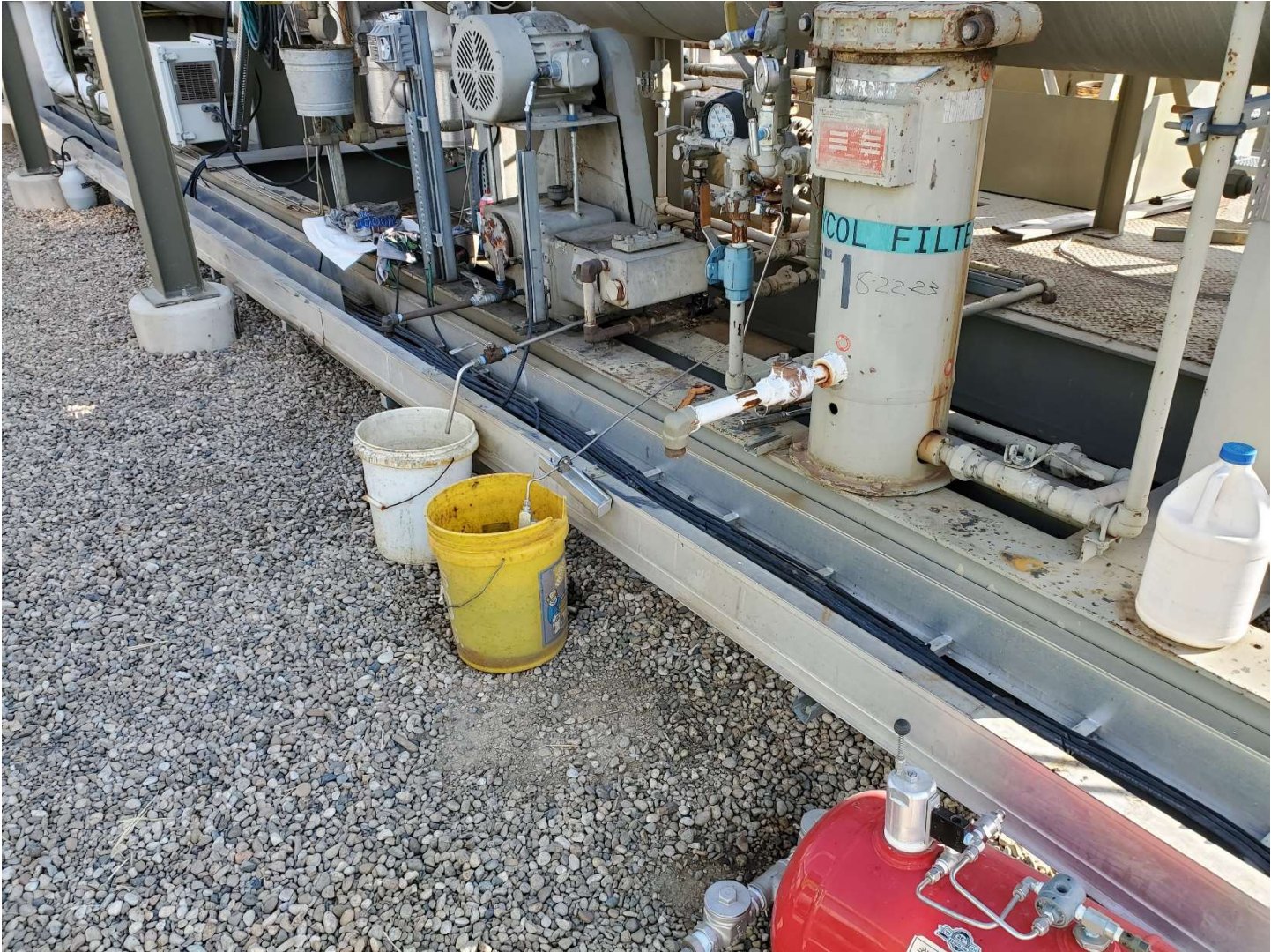
Plastic five-gallon buckets for lubrication spill containment at condensate stabilizer unit.
