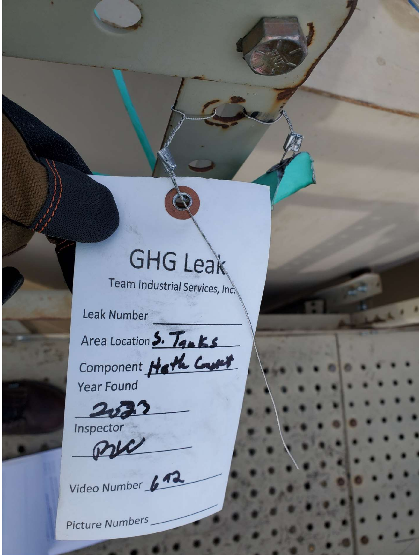
White GHG tag on top of storage tanks.
