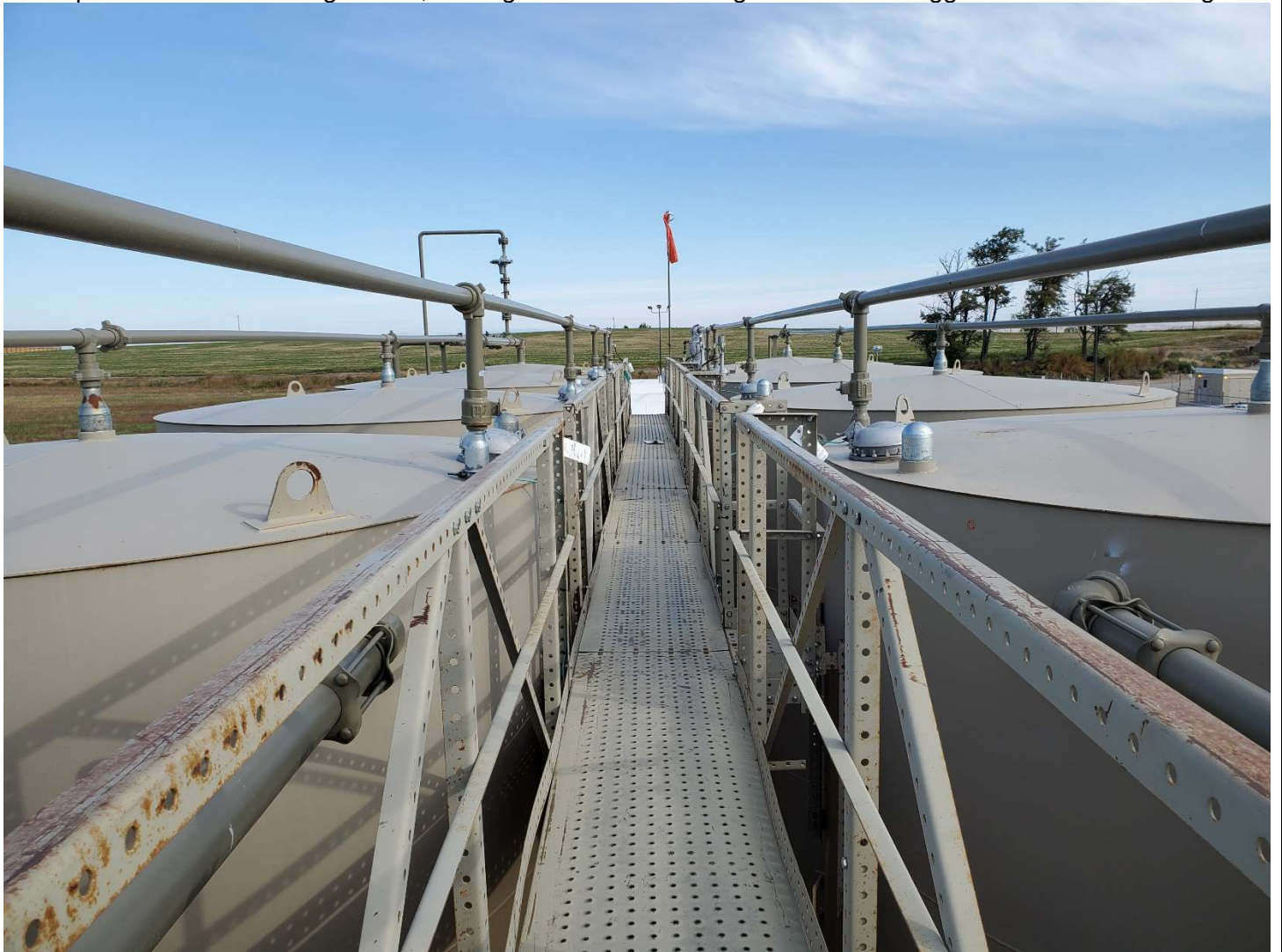
Top of condensate storage tanks, looking north. Seven of eight tanks were tagged with white GHG tags.
