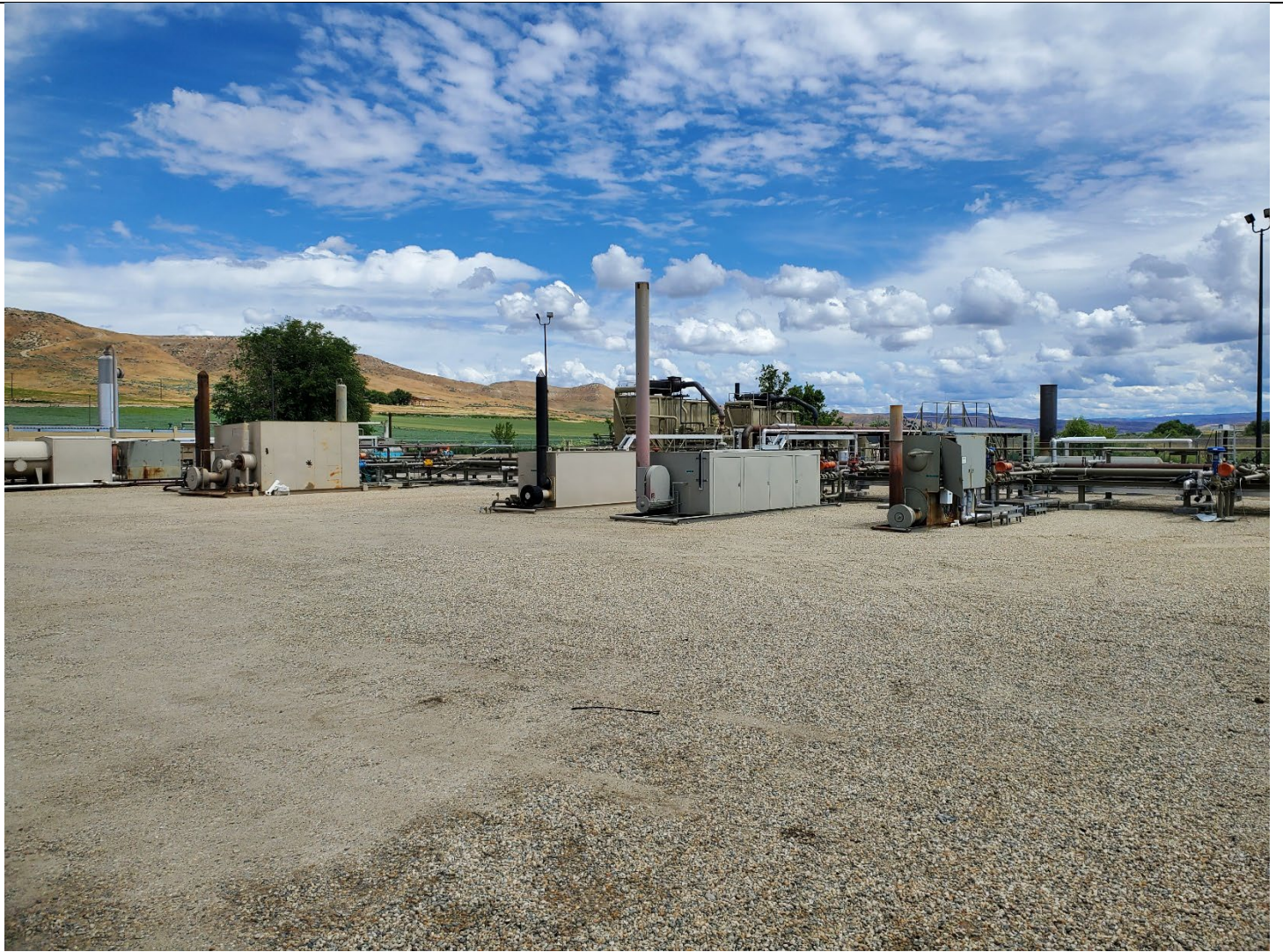
View north of well separator units. From left to right: combined well (Kauffman 1-34, ML 1-3, ML 2-3), ML 3-10, ML 2-10 and ML 1-11 UT. ML 1-11 LT separator has been removed.
