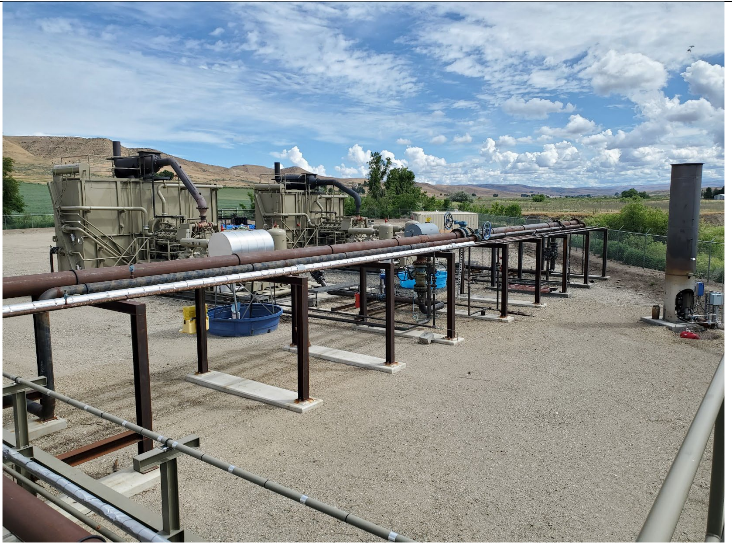
View north of new compressors installed to replace the former single compressor.
