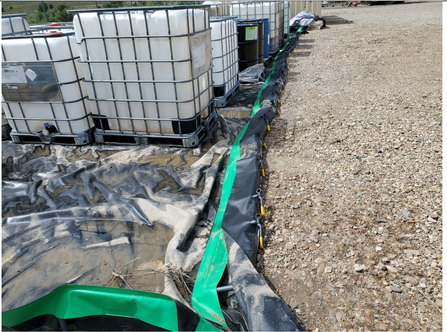
Portable spill containment berm with palletized chemical containers, east side of facility. View is southwest. Spill containment berm is not staked properly and north perimeter is flat.
