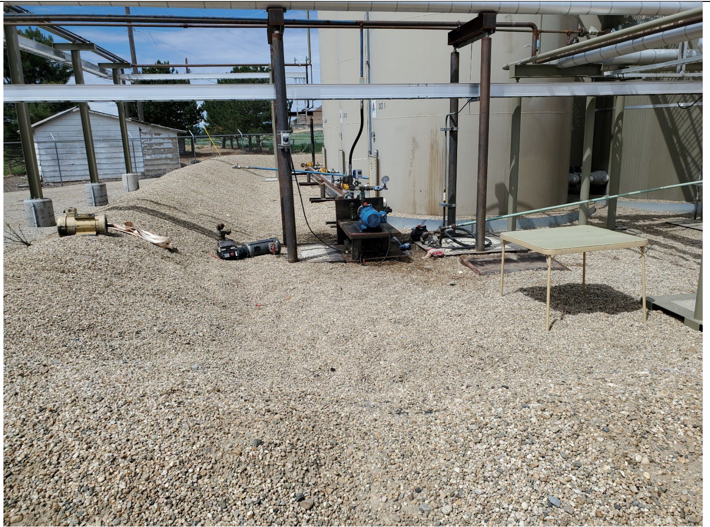
400 barrel produced water tanks and southeast side of containment dike, view southwest. Equipment inside containment dike from recent maintenance and installation operations. Worn foot paths over the dike indicates the access ladders are not being fully utilized and the liner is exposed in multiple areas on both dikes.
