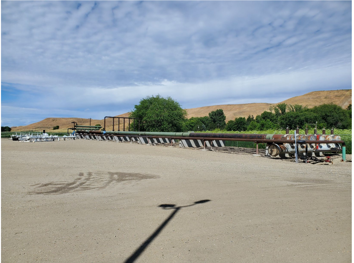
View west of 6-finger slug catcher with gathering system riser on left.
