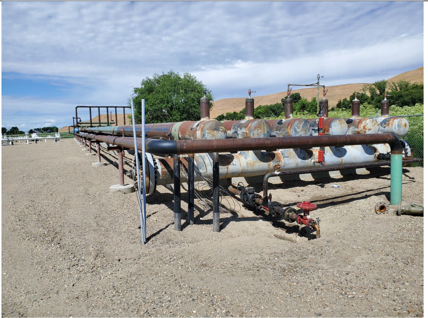
Detailed view of east side of 6-finger slug catcher, looking west.
