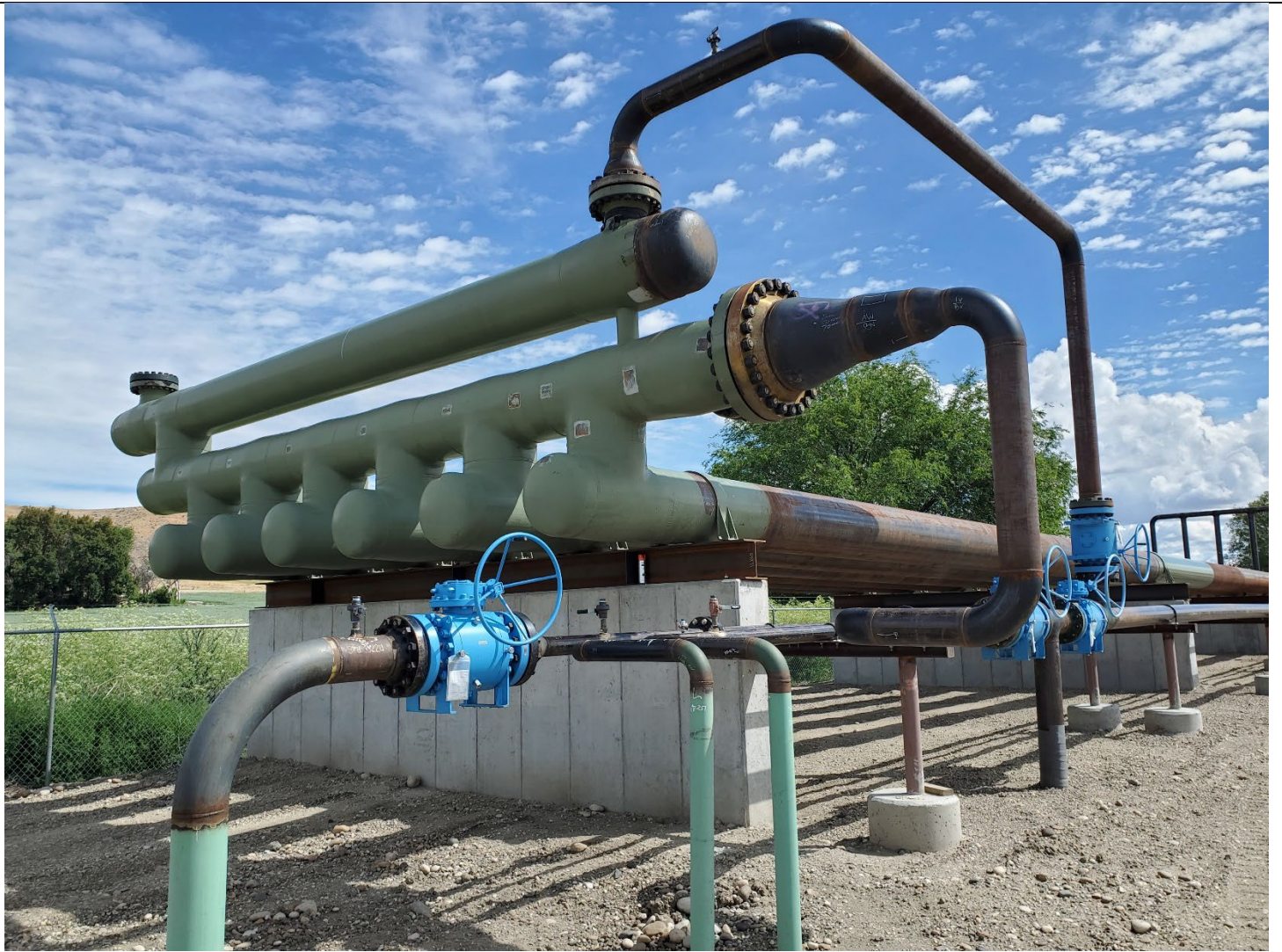
Detailed view of west side of 6-finger slug catcher, looking north.
