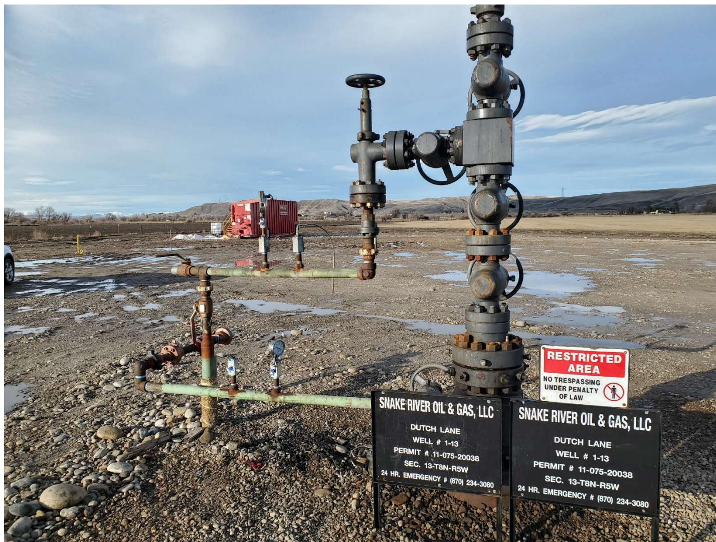
Wellhead with temporary water tank, north side of wellpad. View north 1/12/2023.
