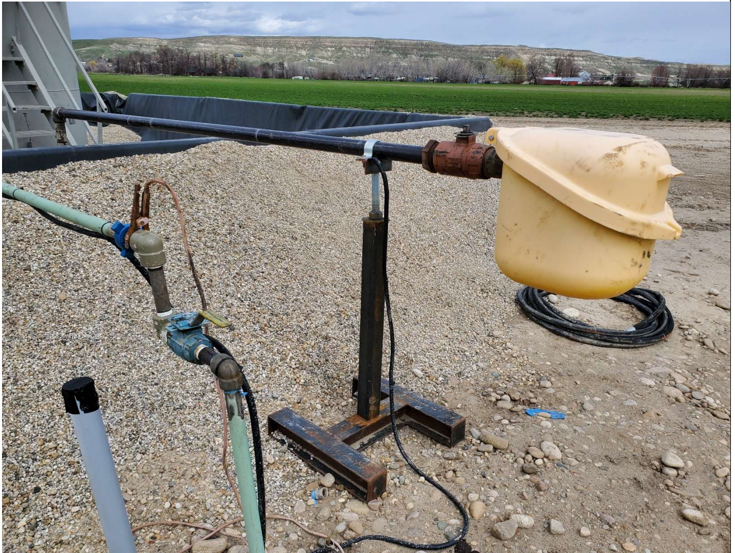
Detail of water intake line from separator, quick coupler and spill containment device on south side of containment dike. View is northeast 4/12/2023.
