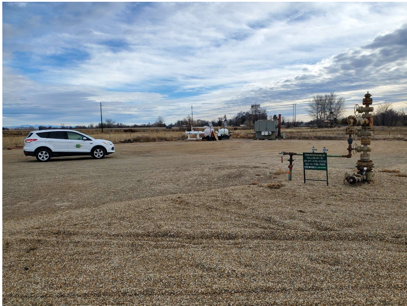
Well head, separator and gathering line riser, view southeast 1/12/2023
