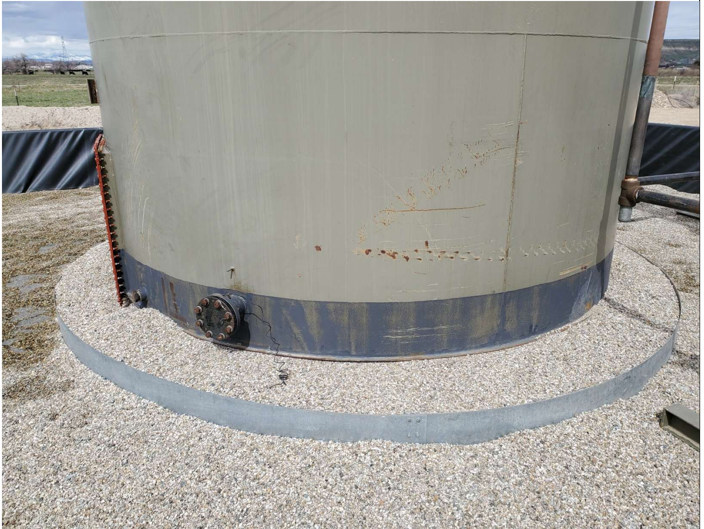
Detail view of the gravel base installed to support the 400-barrel tank within the containment dike. View is northeast.
