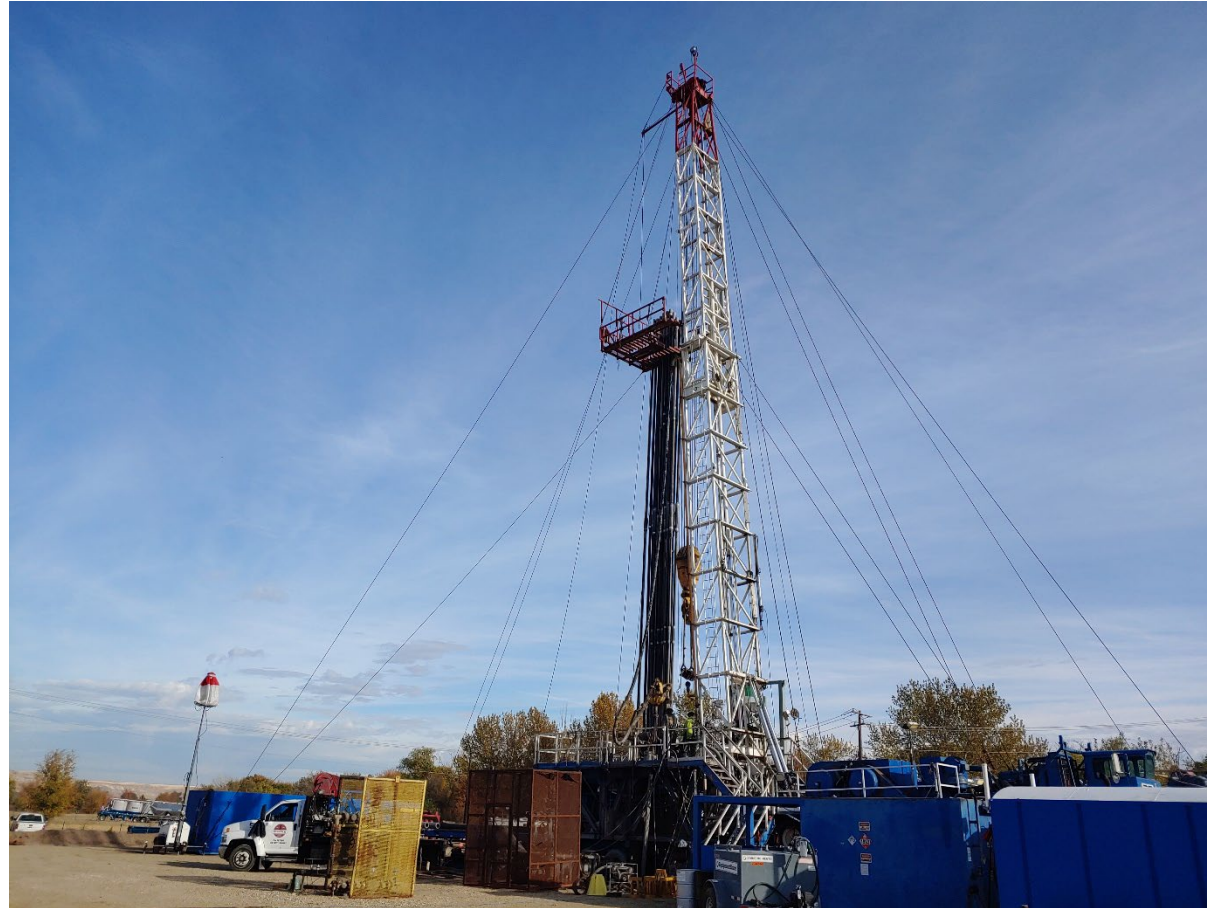
GRAHAM #4 RIG ON SITE FOR DRILLING OPERATIONS ON THE BARLOW #3-14, HARMON FIELD, PAYETTE CO. ID. OCTOBER 2022 PHOTO COURTESY J. THUM
