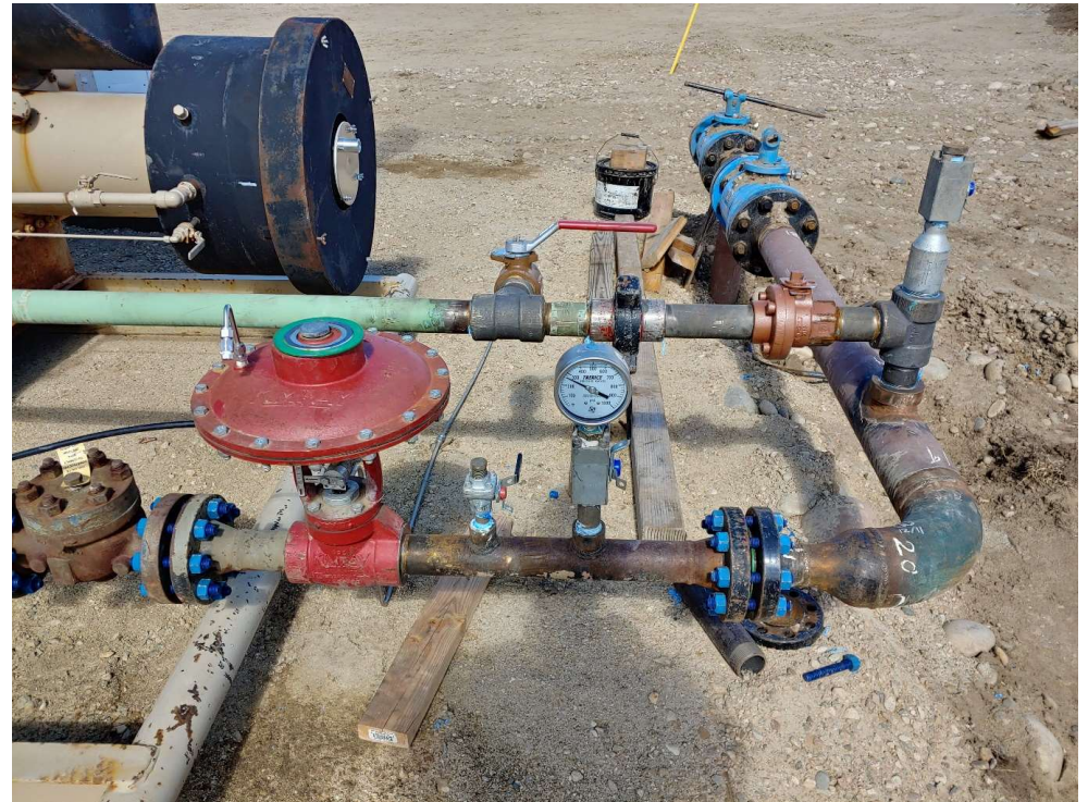
FALLON #1-11 FLOW LINES FROM SEPARATOR UNIT SEPTEMBER 2022 ANNUAL WELL INSPECTION PHOTO COURTESY J. THUM
