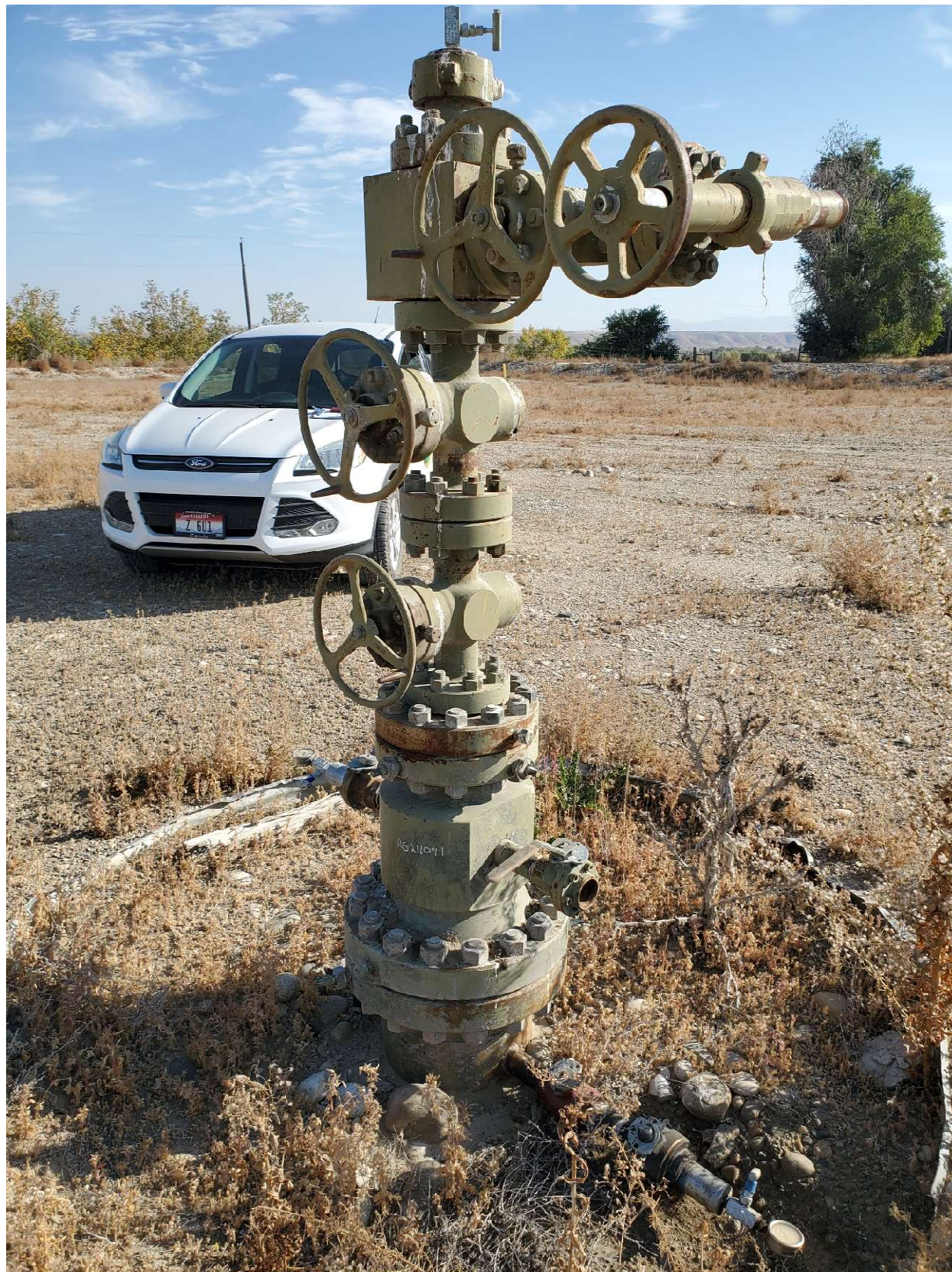
Wellhead, view NE, Note weed encroachment in cellar and east side of well pad/
