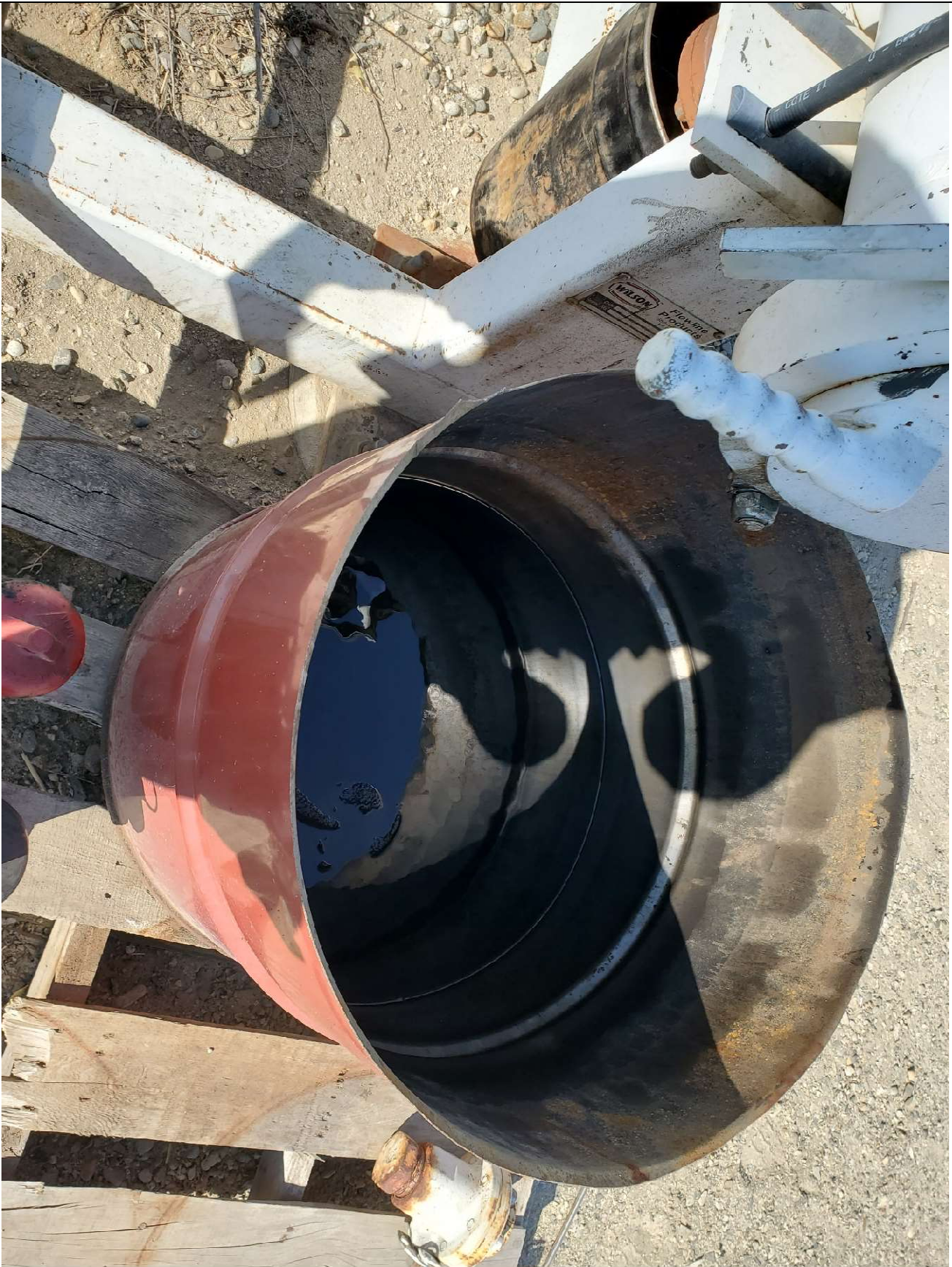
Chemicals outside of portable spill containment device, NW side of facility. Ripped containment device, center of photo.
