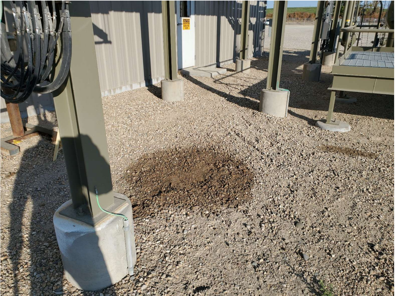
Spill stain on gravel, east side of compressor building.
