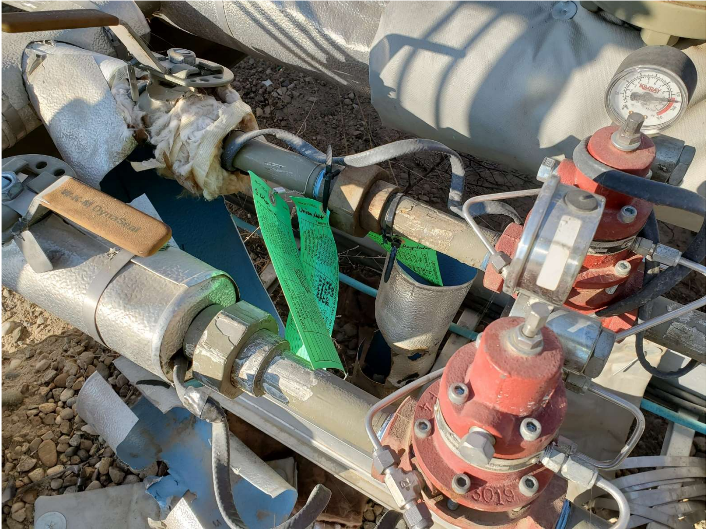
Condensate / NGL flow line repair tags, SW side of facility.
