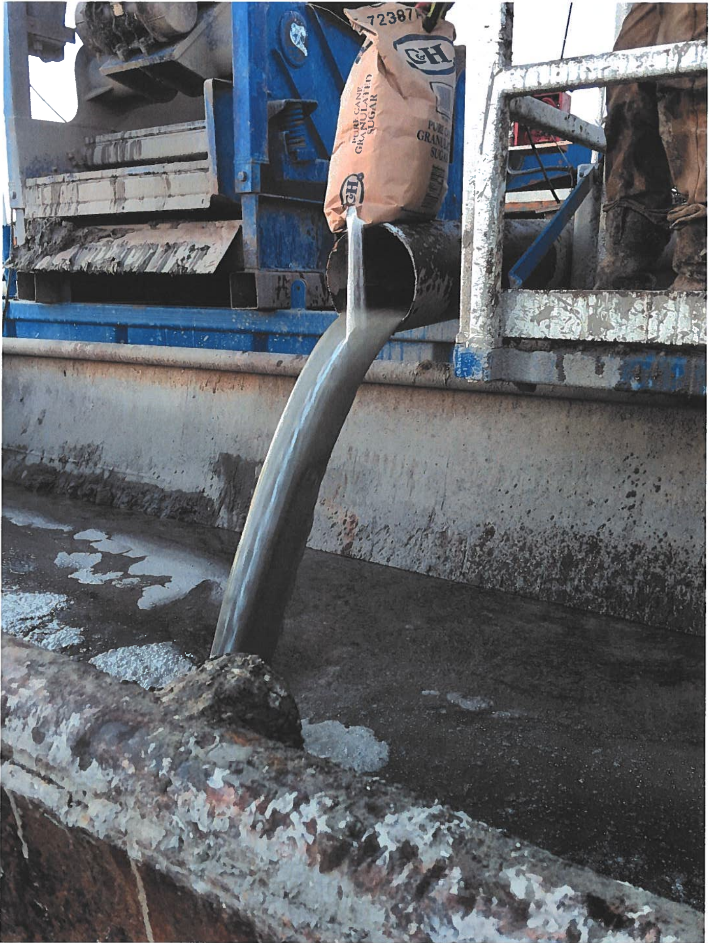
Cement Returns during cementing of surface casing of Irvin 1-19. Estimated 85 barrels of cement returns.
