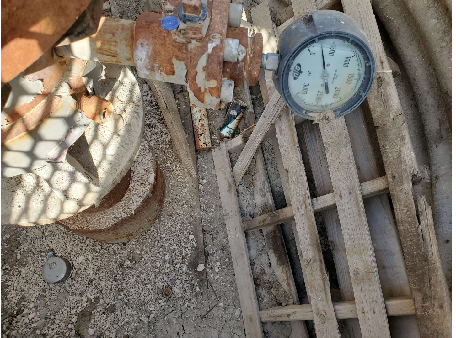
View of wellhead cellar showing pallets and other debris around surface casing.
