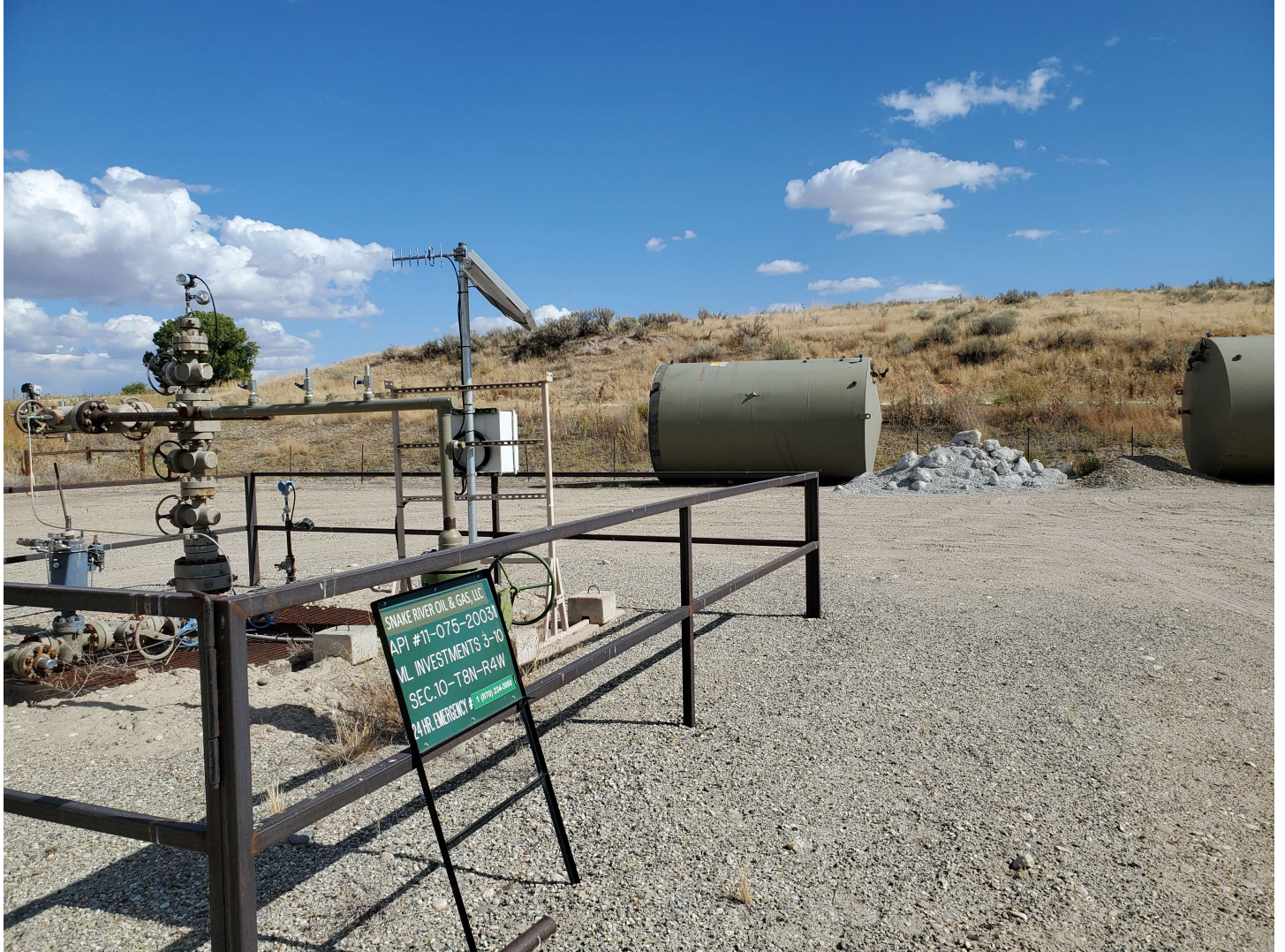
Wellhead view looking SE. 400 bbl storage tanks being stored on site along SE perimeter of well pad.
