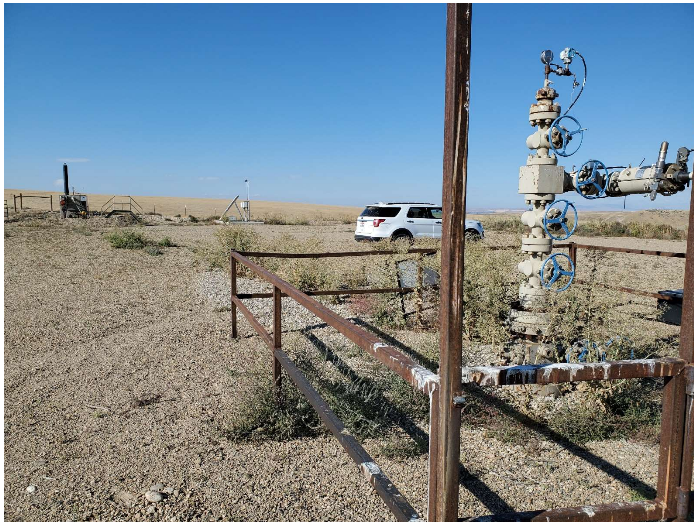
Well head right foreground, separator unit and SCADA transmitter left background
