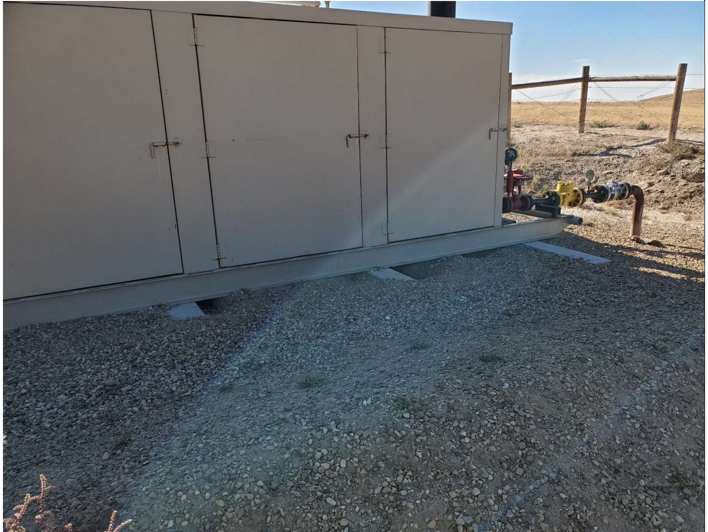
Separator unit showing signs of animal excavation under and around support footings.
