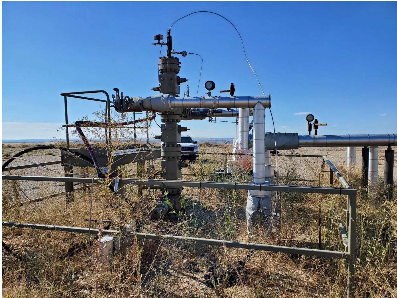
Well head and steel protection fence showing extensive weed encroachment. View is south.
