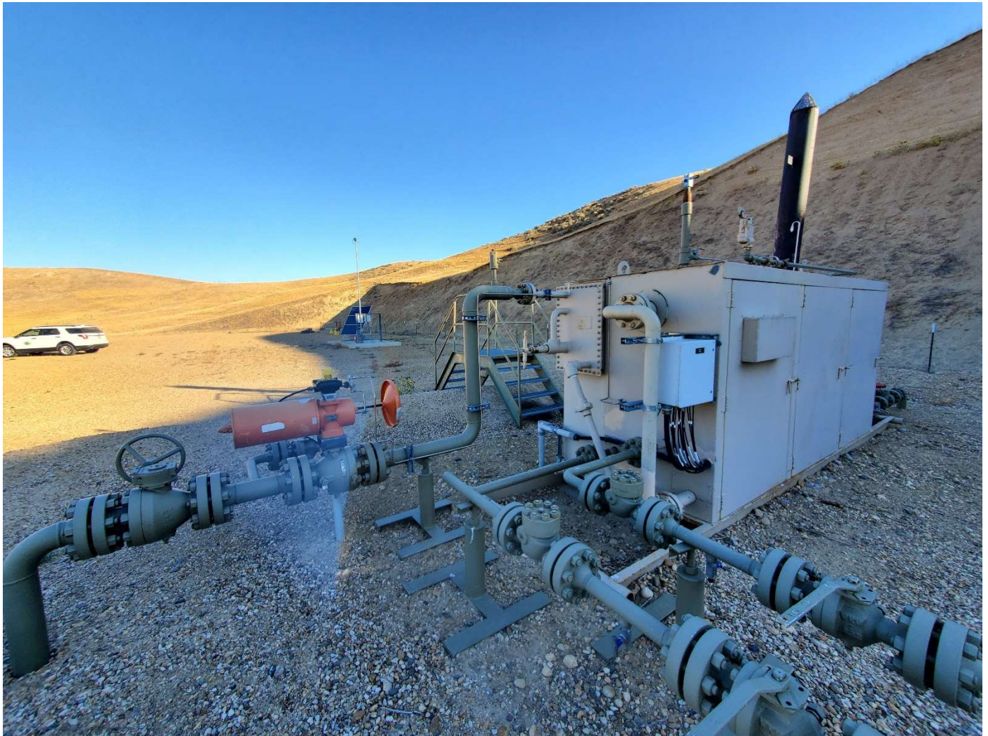
Separator unit with SCADA remote in background.
