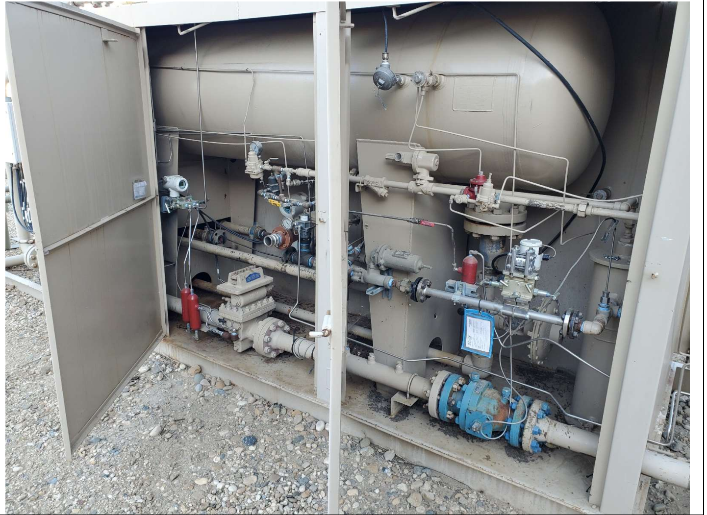
Inside separator unit housing.
