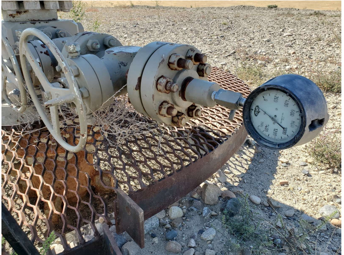
Detail of well head, surface casing gauge and cellar (no water nor debris present).
