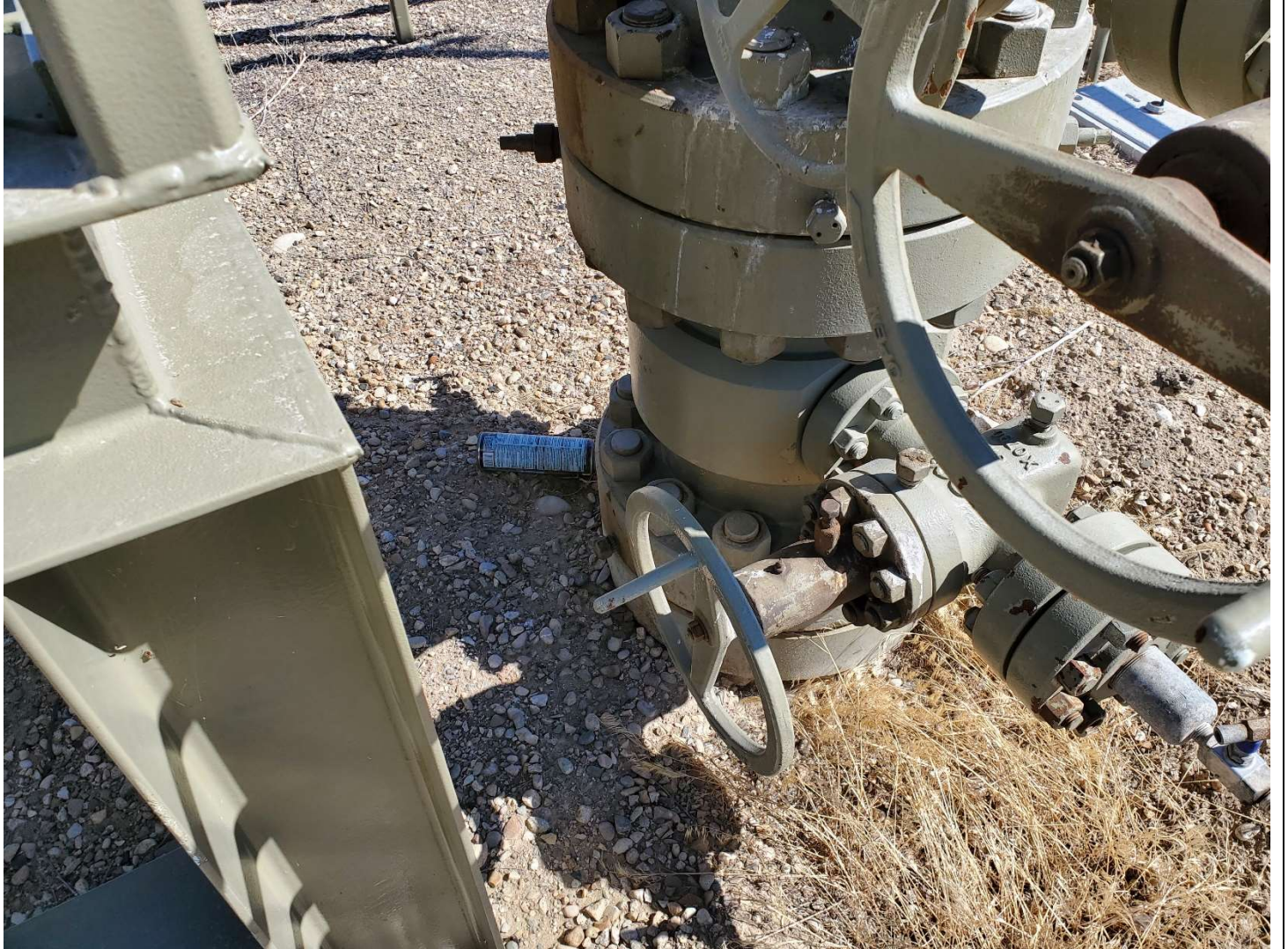
Base of well head with gravel filled cellar.
