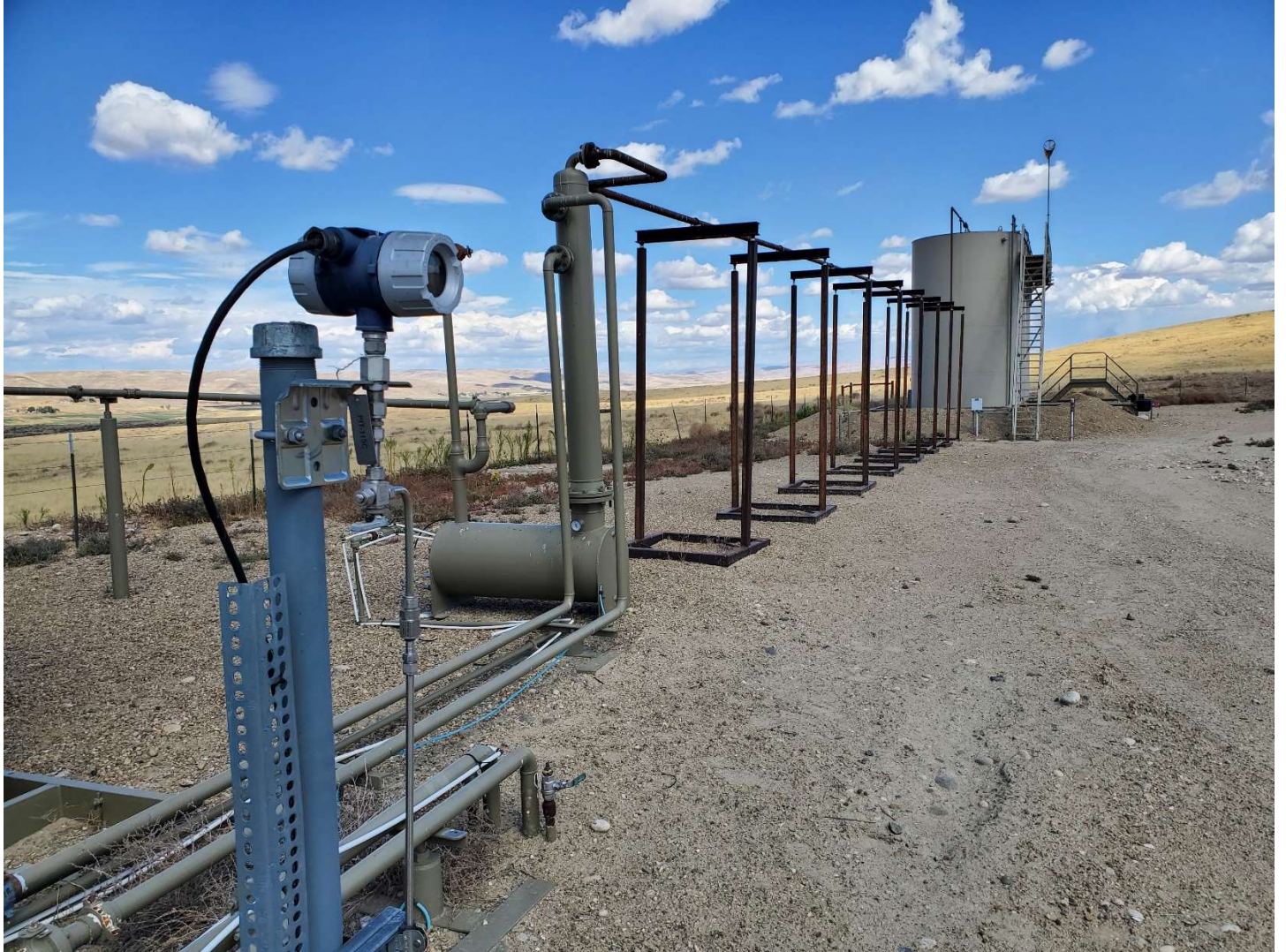
Northwest perimeter of well pad, produced water tank batter in background, view NE. Note weed encroachment along fence and tank battery dike perimeters.
