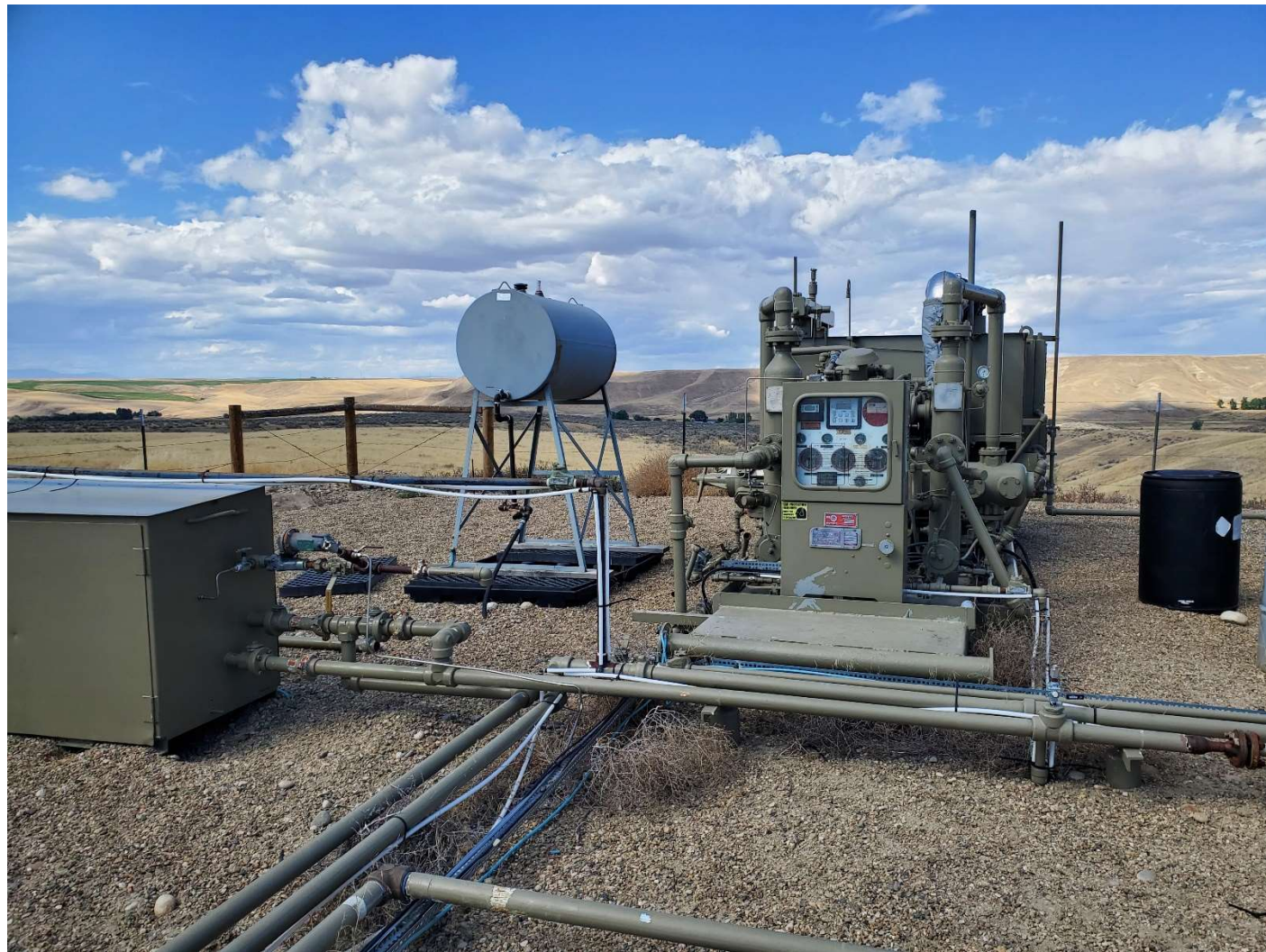
Separator unit in west corner of well pad, view west.
