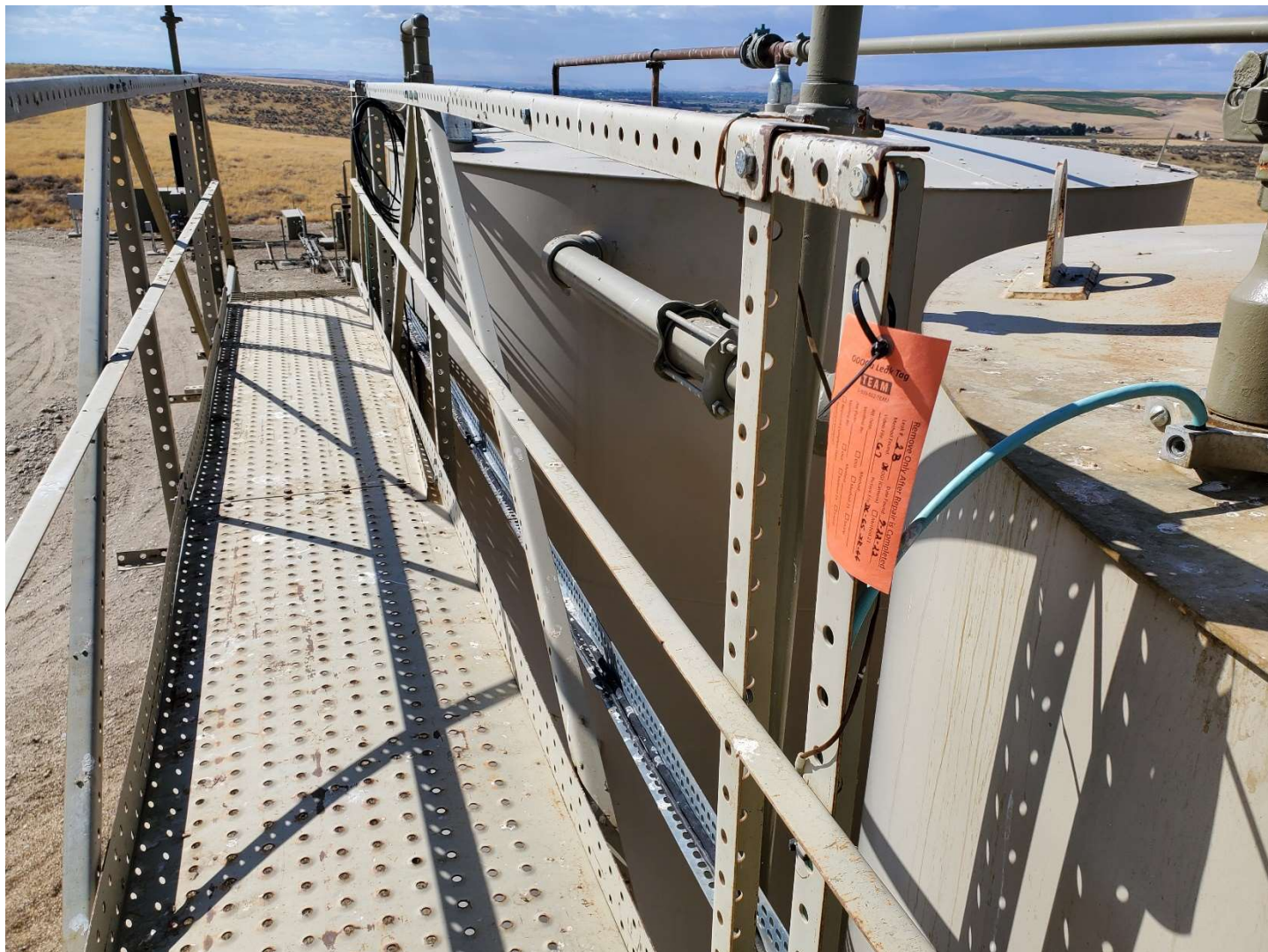
View SW of tank battery from the top, leak detection hang tag for middle produced water tank.
