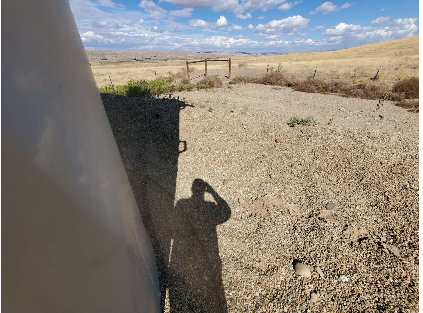
NW corner of containment dike, view N. Note livestock disturbance on and within tank dike.
