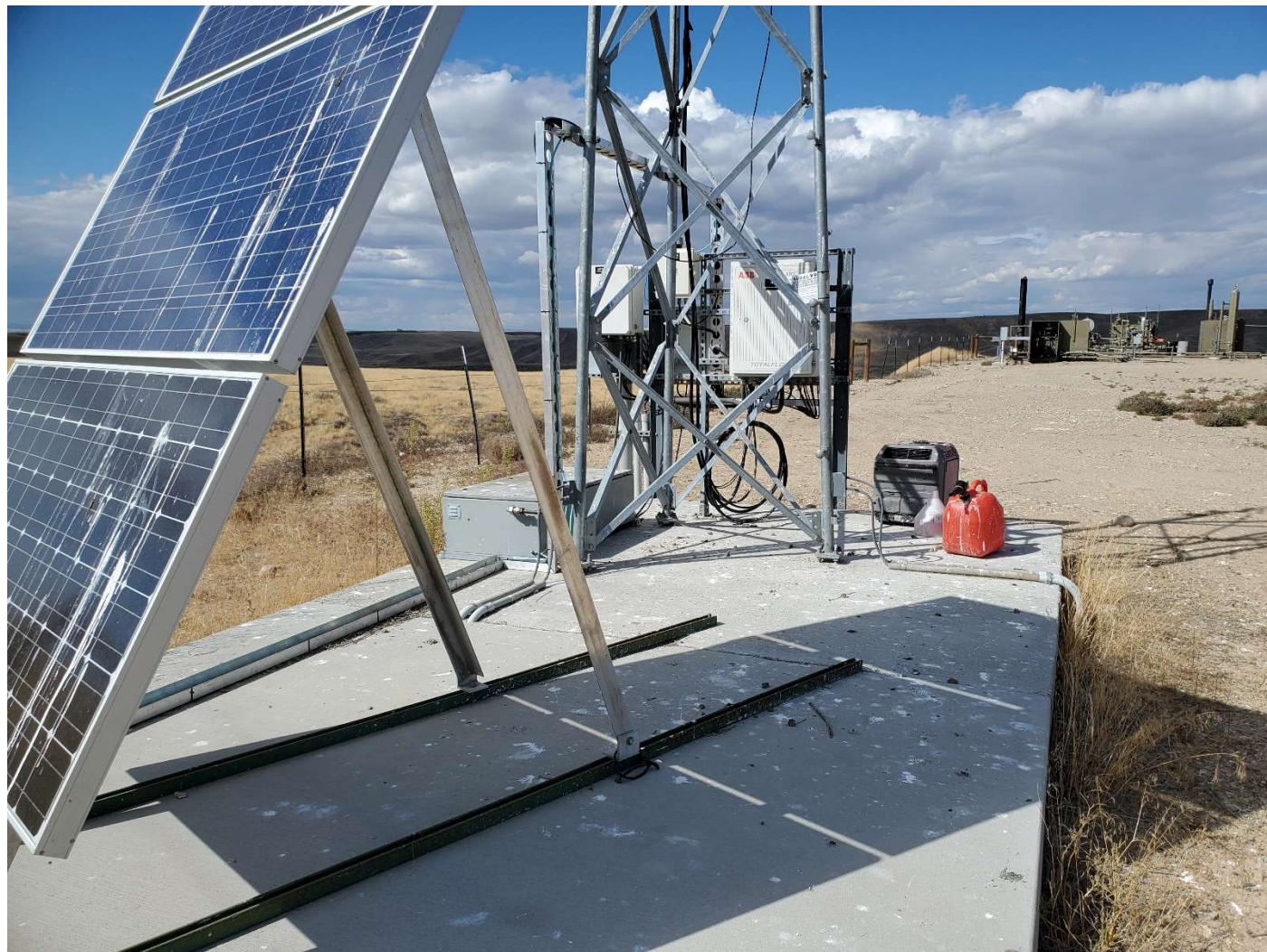
Pad for communications tower, south corner of well pad, view NW. Separator Unit in background right. Generator and gas can sitting on tower pad.
