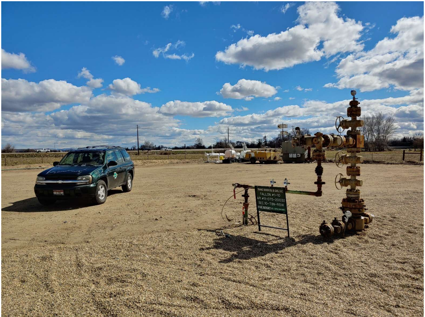
Fallon 1-10 wellhead and sign. Pipeline riser / pig launcher, separator unit and temporary heating unit in background. View SE to US 95.
