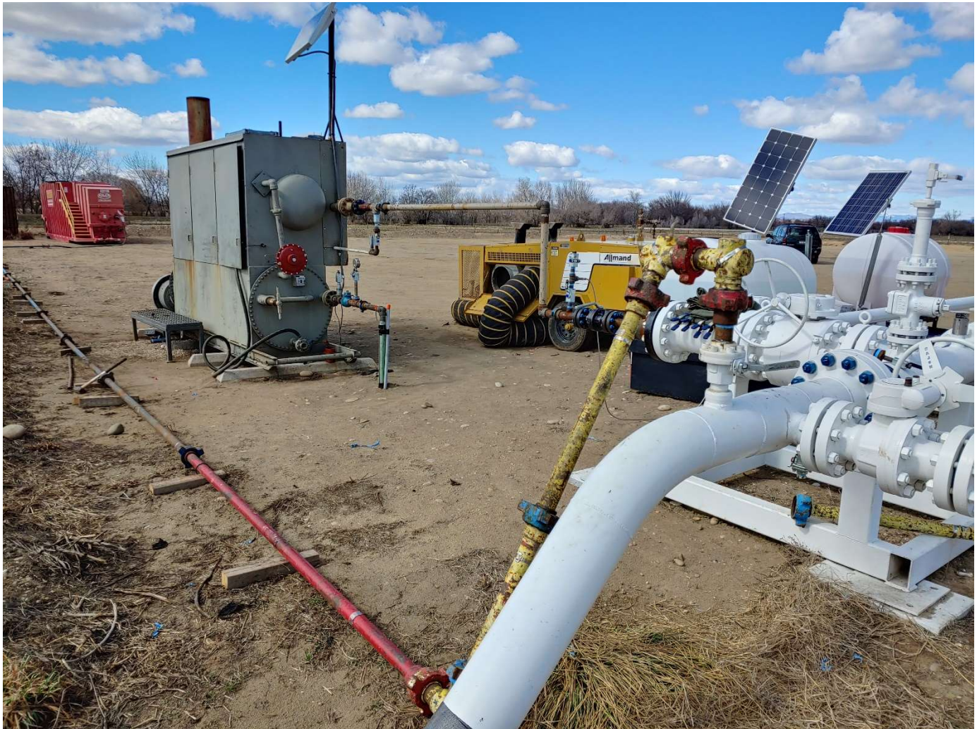
Fallon 1-10 well pad from SE corner, looking NW. Left to right: red temporary H2O tank, gray well separator unit, yellow temporary / portable heating unit, white pipeline riser. Yellow & red surface flow line connected to temporary H2O unit along southern pad dike.
