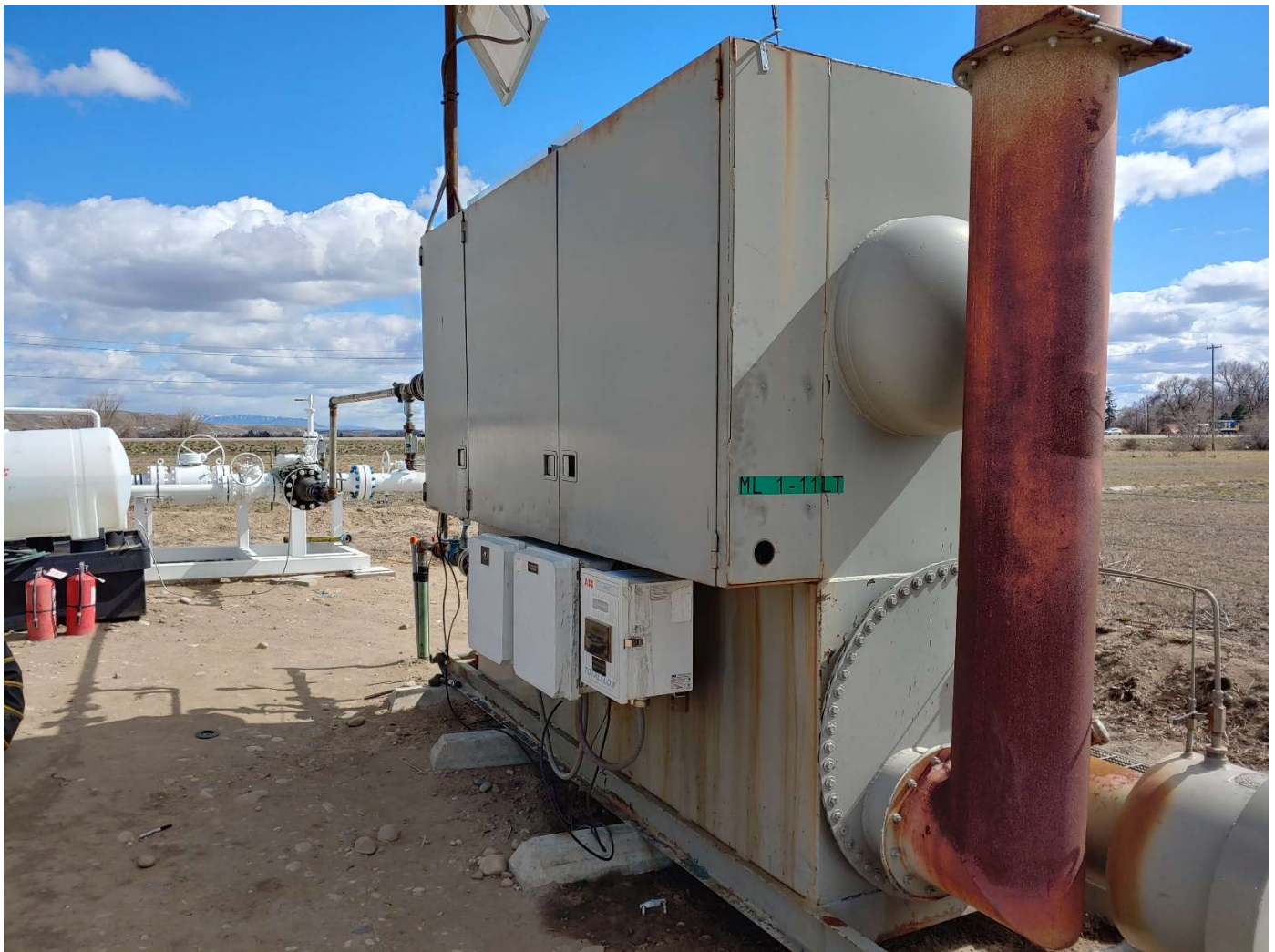
Re-purposed separator unit (mis-labeled as “ML 1-11 LT”) and flare stack, looking East.
