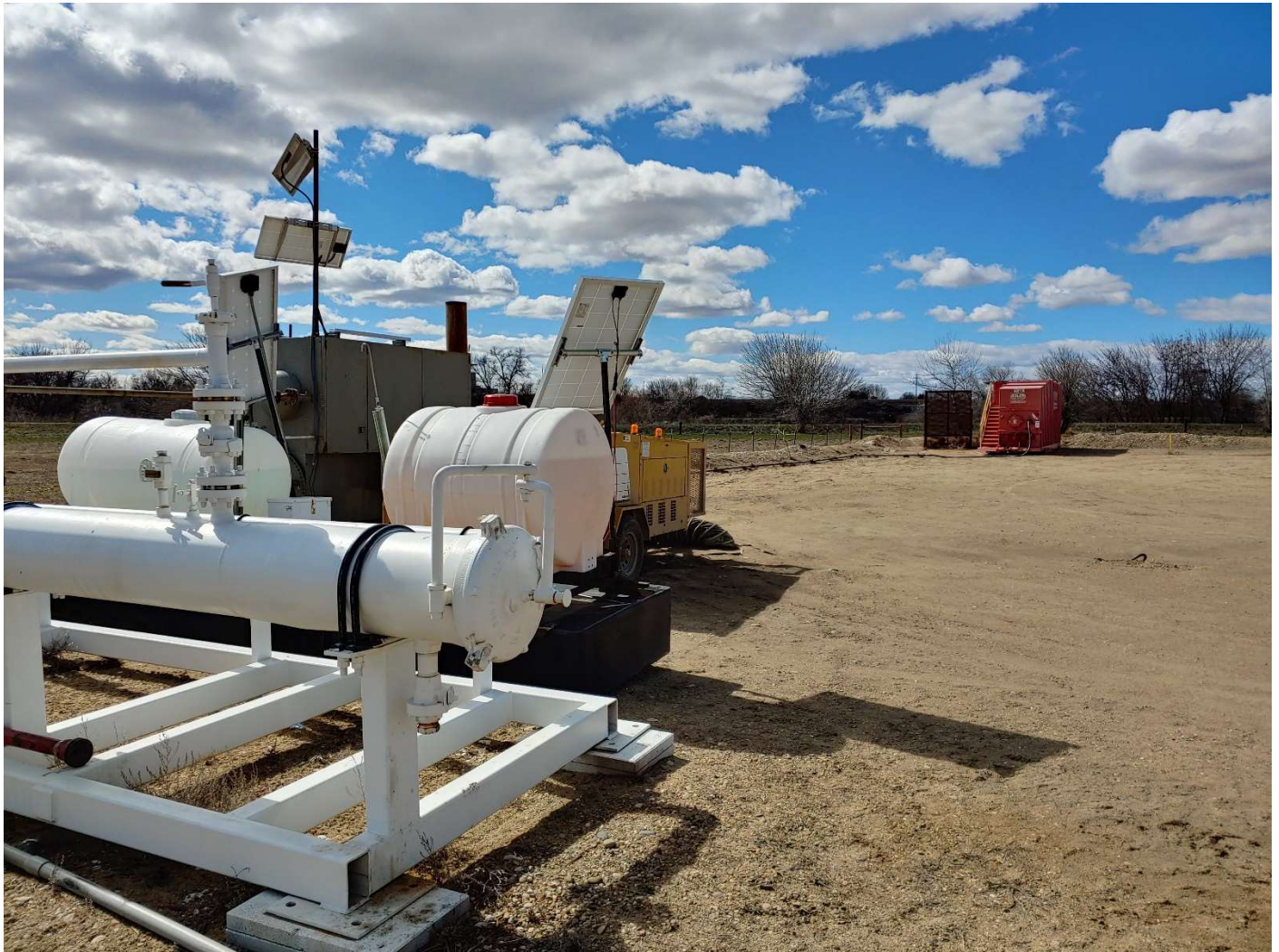
Pig launcher in pipeline riser, separator unit and portable heating unit in background, temporary water tank at right-rear of photo. Phot taken from east side of well pad looking WSW toards SW corner.
