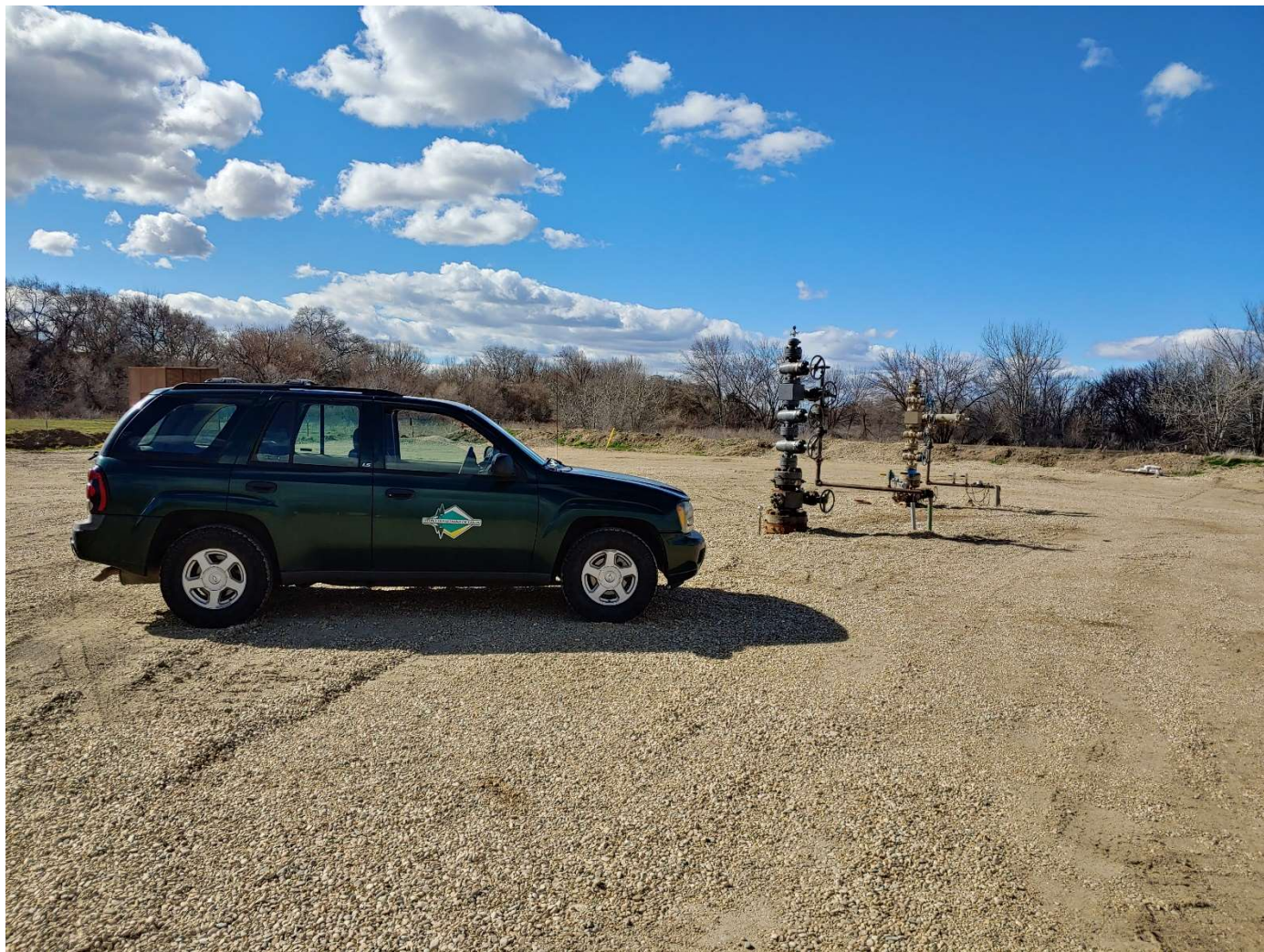
Barlow #2-14 wellhead on the left, Barlow #1-14 wellhead on the right. View NW.
