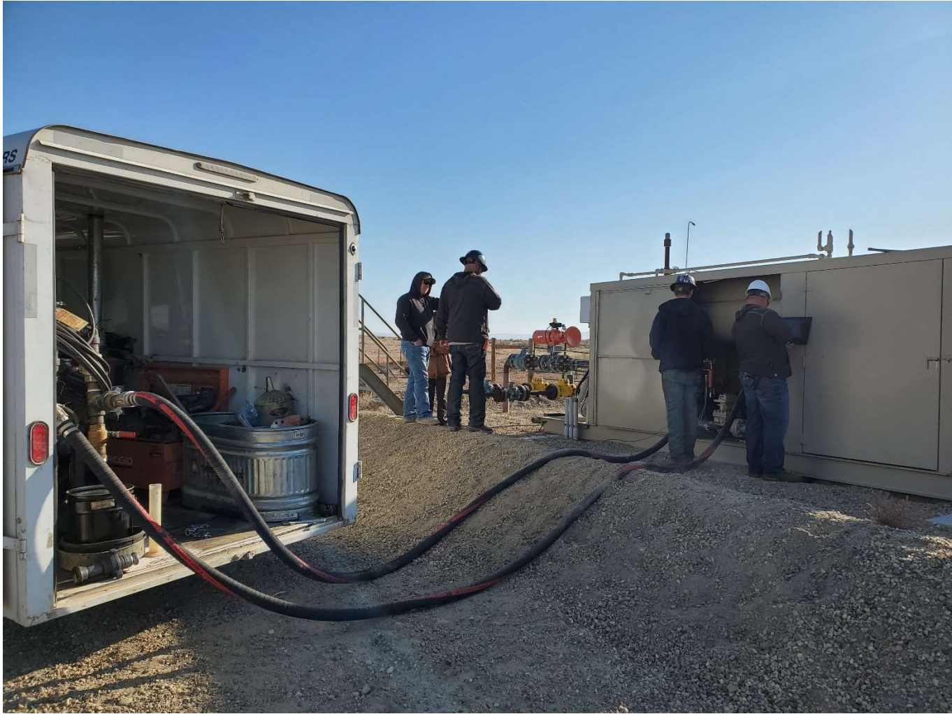
6. SPL meter proving set-up 10/19/2021. Separator/meter housing at right, proving monitors in trailer at left.
