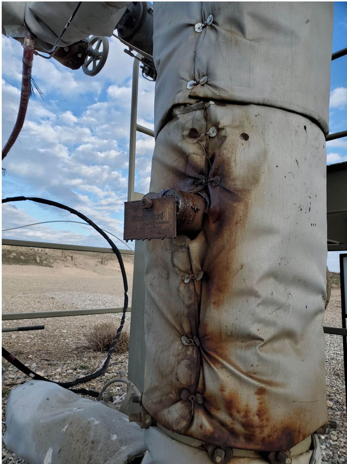
6. Detail of lower wellhead and insulation, view E. Note oil stained insulation and valve stems.
