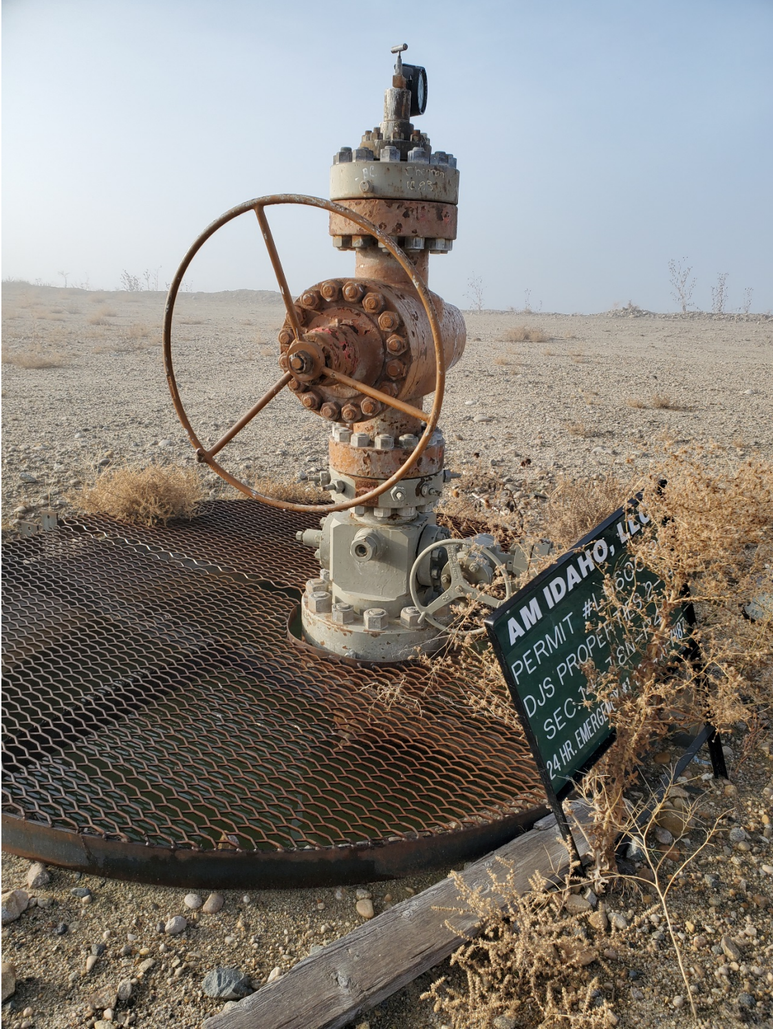
1. Wellhead and cellar, view SSE with incorrect identification sign.
