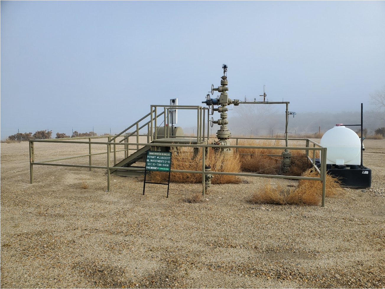
1. Inner wellhead fencing looking ENE with chemical storage tank on right.
