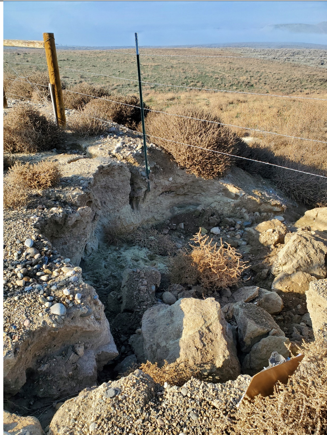
Pad erosion looking WNW from NW corner of tank dike. Note suspended fence stake.
