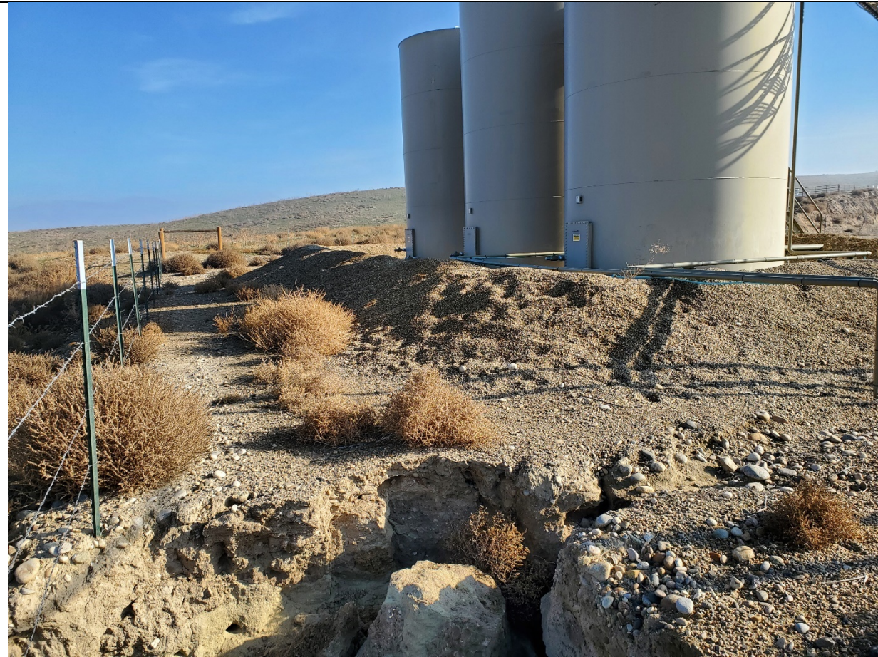
Tank battery and tank dike, North perimeter looking NE. Note pad erosion in lower foreground.
