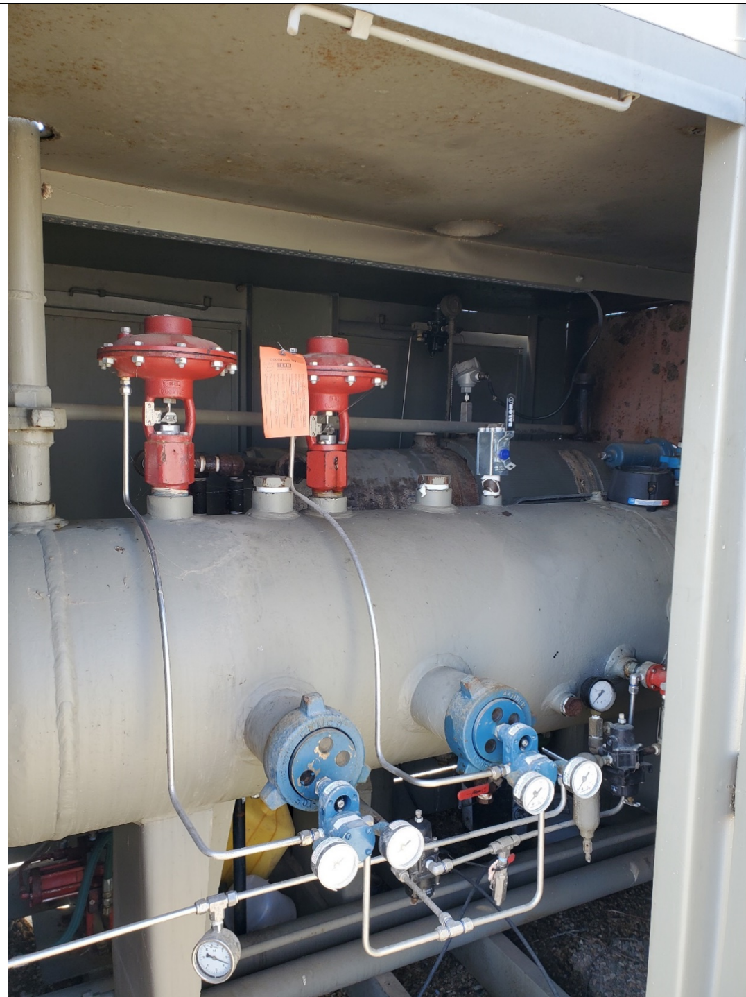
Inside Separator Unit, note orange leak tag.
