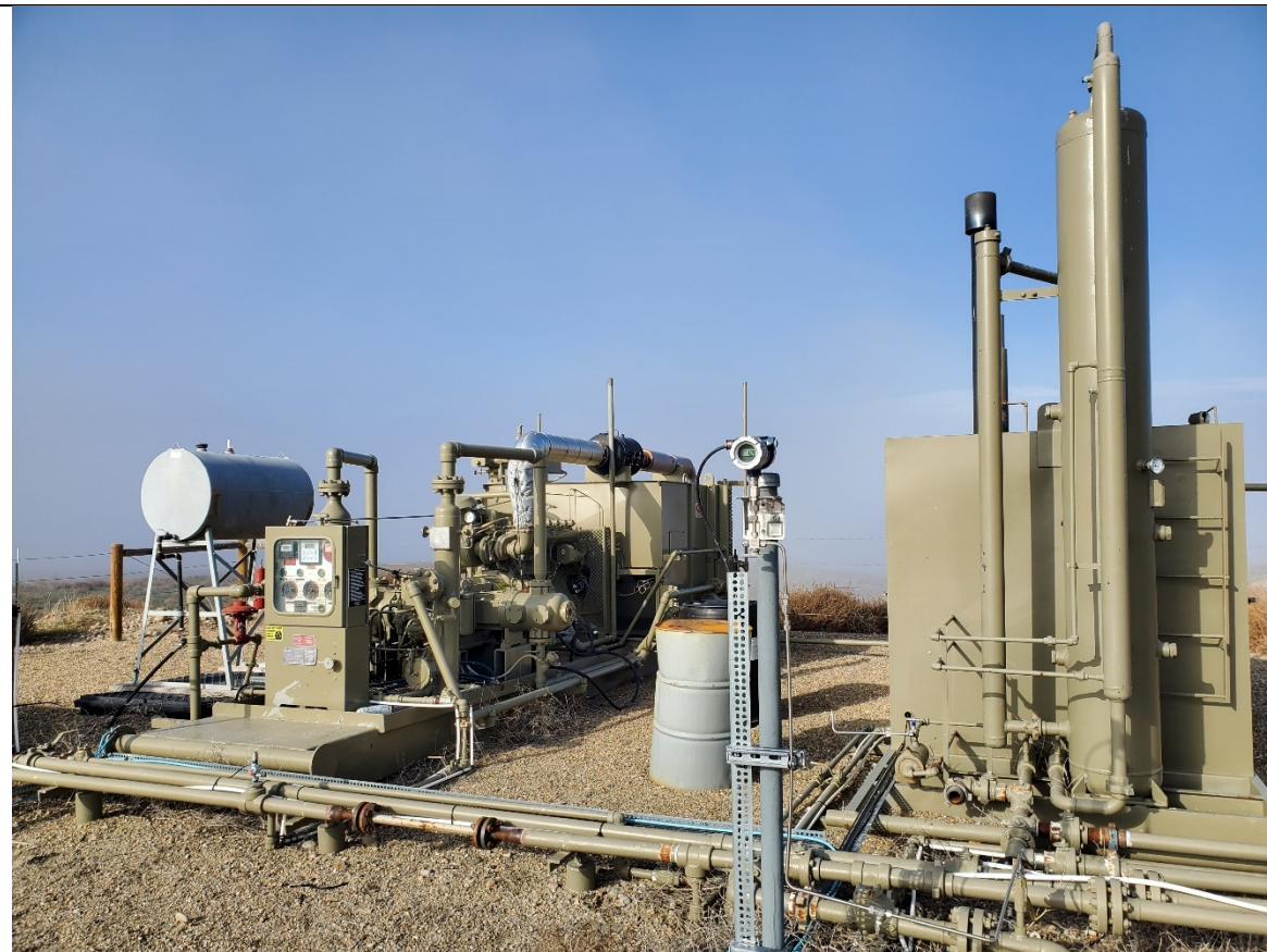
Compressor Unit (right), Separator (left)
