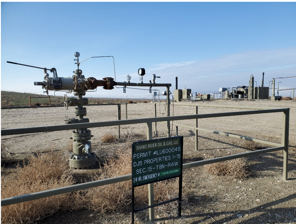
Close-up of well head looking WNW showing well identification sign, separator and meters back right.
