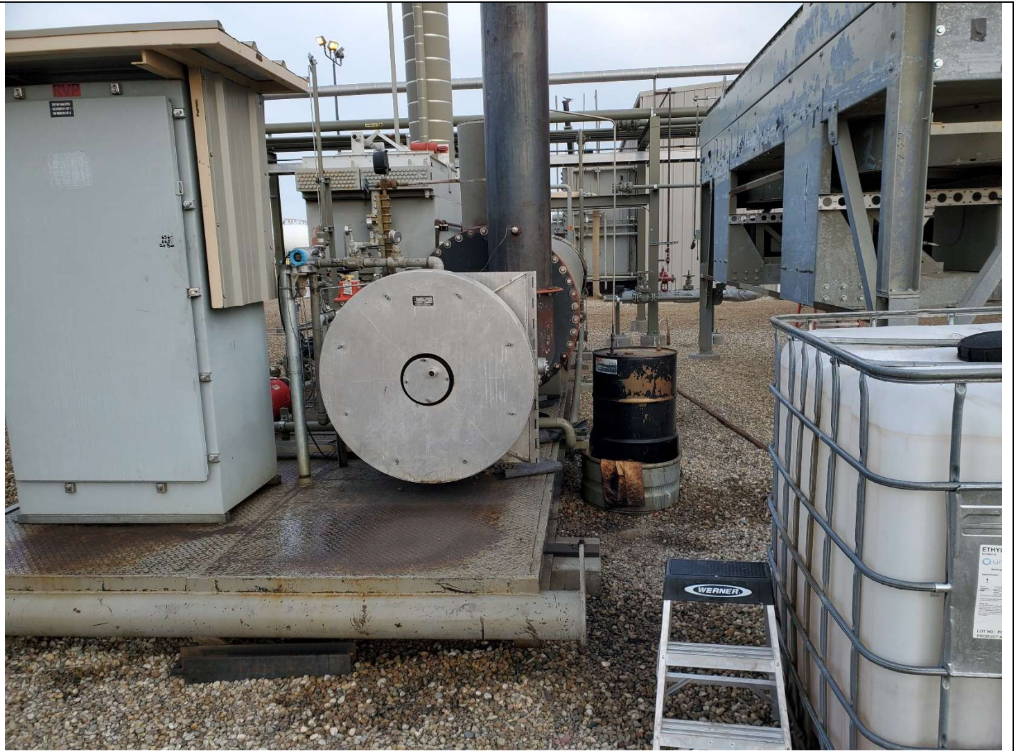
Condenser Unit, looking North. Apparent gravel staining from maintenance operations. No leaks visible at time of inspection. Minor clean-up needed.
