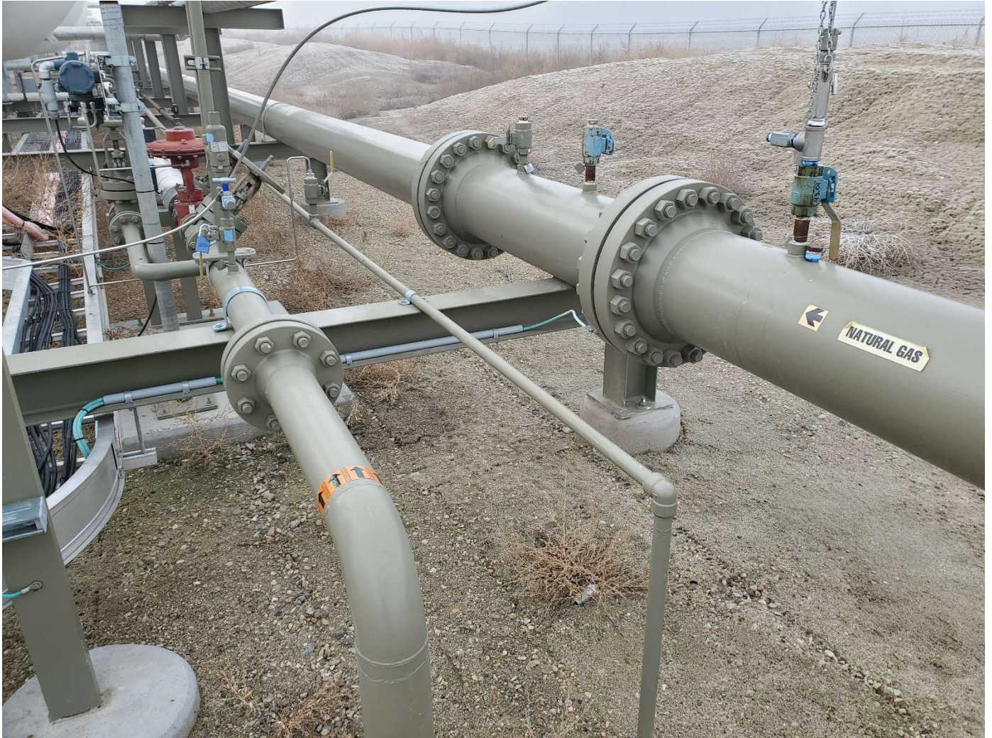
Intake pipeline, west side of Highway 30 facility looking SW. Some vegetation present.
