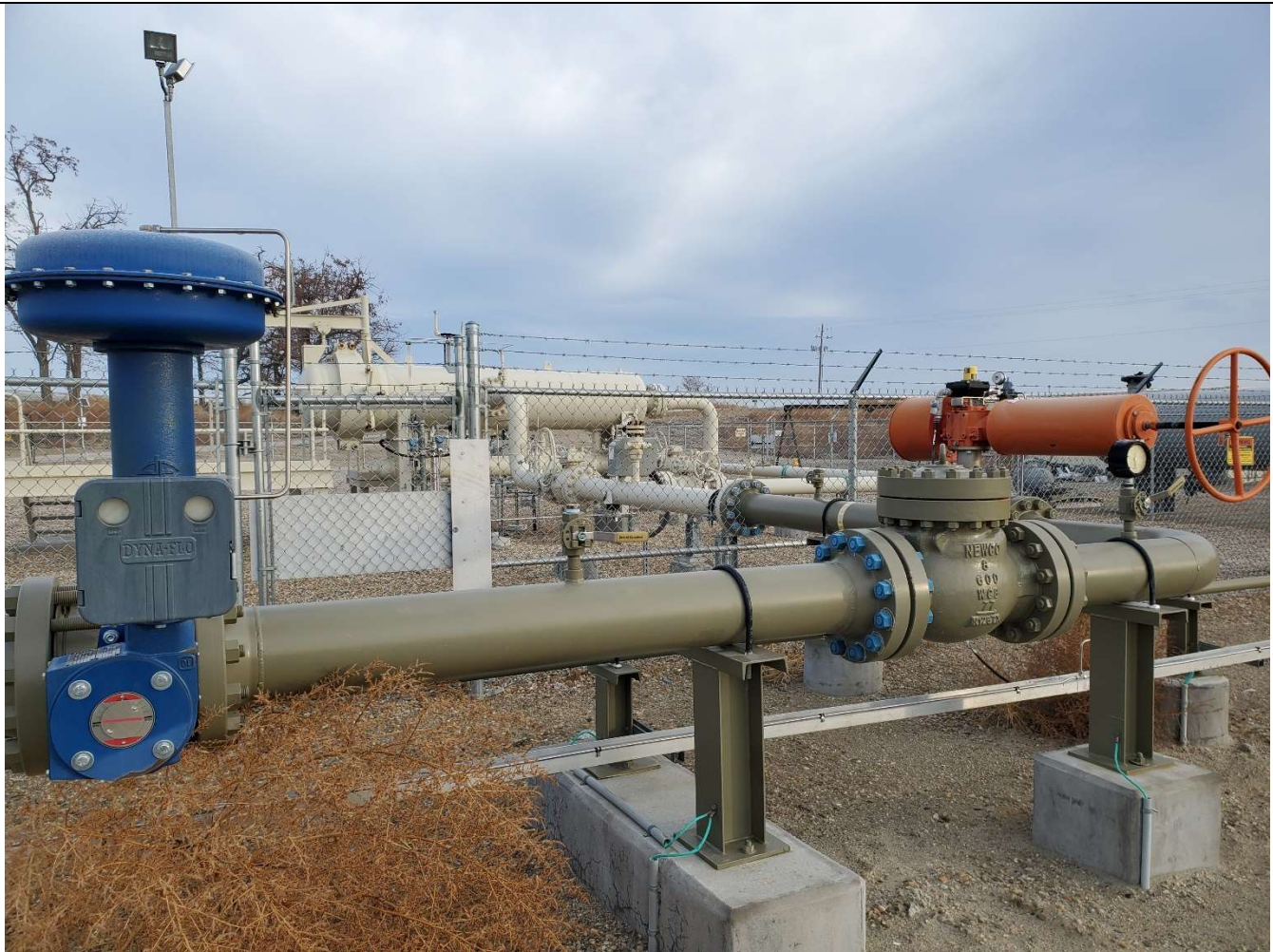
Highway 30 to Williams Pipeline tailgate looking NNE. Additional vegetation remediation needed. Equipment all in good shape at time of inspection.
