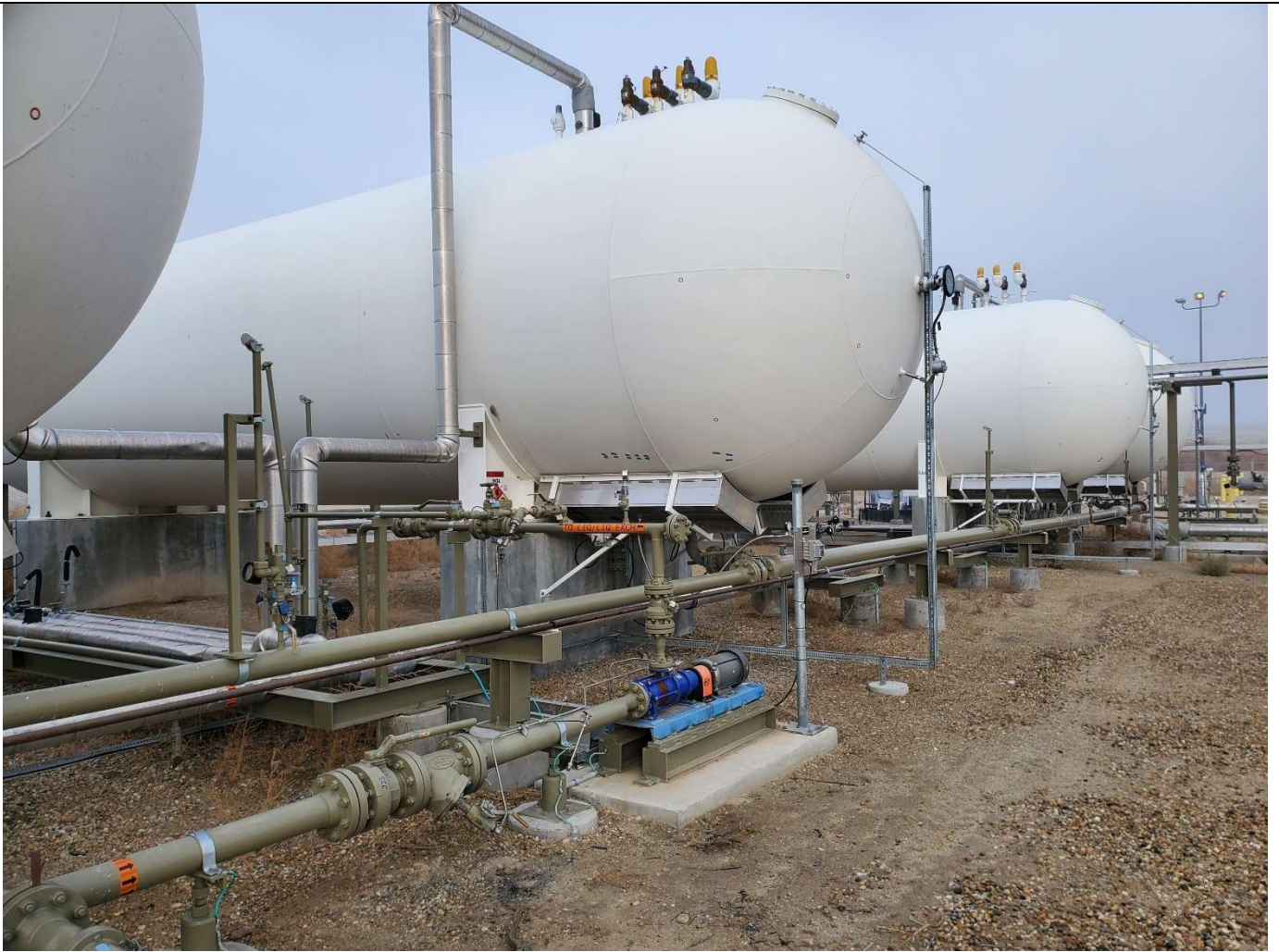
NGL storage tanks, looking NW. Some vegetation abatement needed. Otherwise everything is in good shape.
