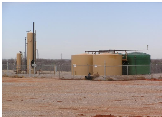
Figure 4-18 Tank battery in northwest Oklahoma City - Source, GWPC
